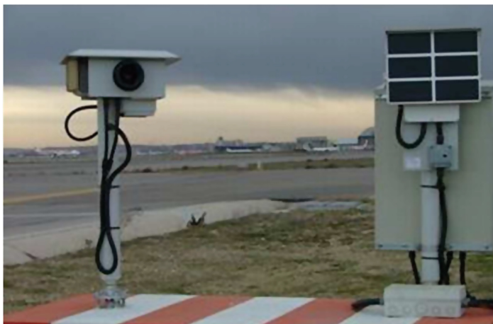
Fig. 3. OIS sensor in apron T4 of the airport.
