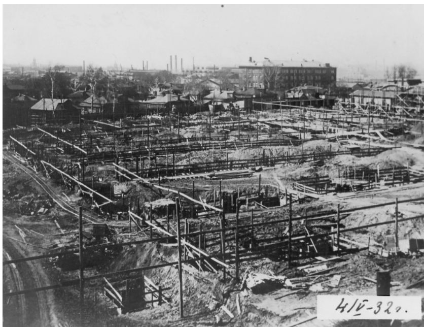
Construction at Serp i Molot (Hammer and Sickle), one of Moscow's largest metallurgical complexes. 1932.
