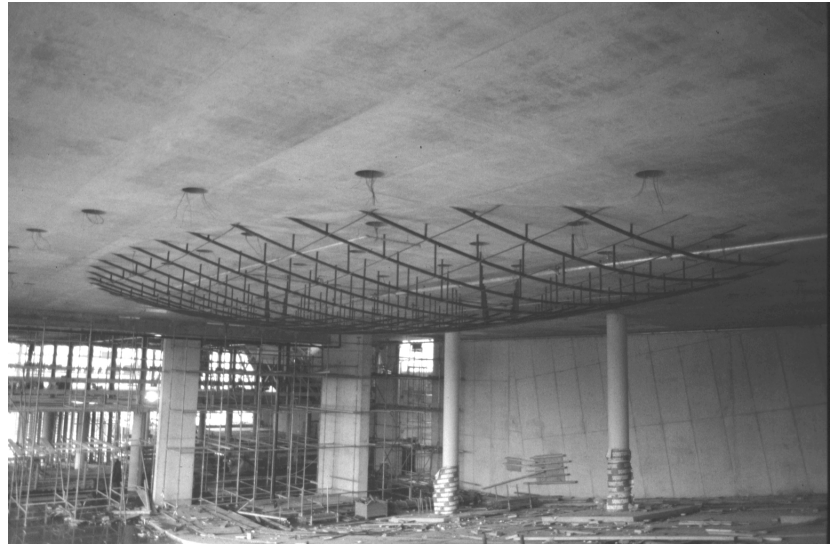
Figure 5-24 The concrete slab with a "belly" of reinforcement hanging out in the middle.
