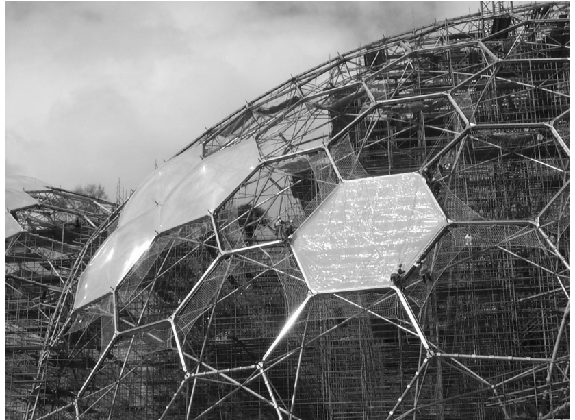
Case 4-18 ETFE cushion, relative ease of construction. (Note the size of the scaffold in the background!)
