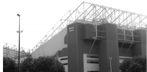
Figure 5-15 The trussed roof is tied to the seating structure at Manchester United.
