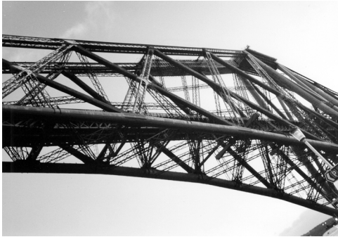
Figure 5-20 The Forth Bridge – there is a clear distinction between the tension and compression members.
