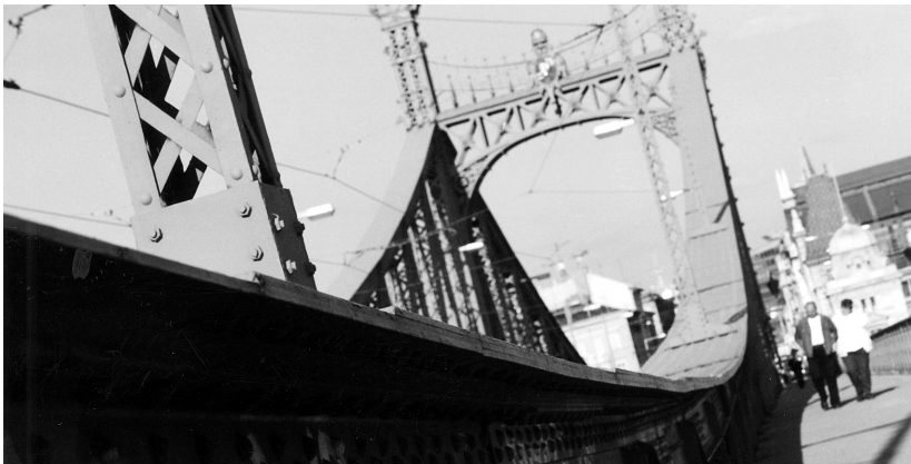
Figure 5-22 The Szabadsag Bridge in Budapest, close-up of the widening and thickening of the top flange of the cantilevered beams.
