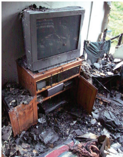
Figure 5.42. Photograph of damage from a candle-ignited fire that destroyed a campus fraternity house in Amherst, MA. Flame retardants likely prevented the television and surface-treated wood cabinet from igniting. Reproduced from http://www.buildinggreen.com .
