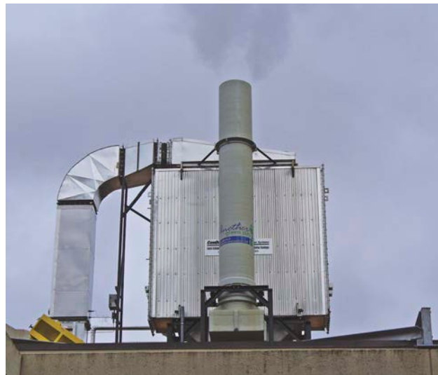
Figure 7.51 Boiler heat recovery system. Source: Providence St. Peter
