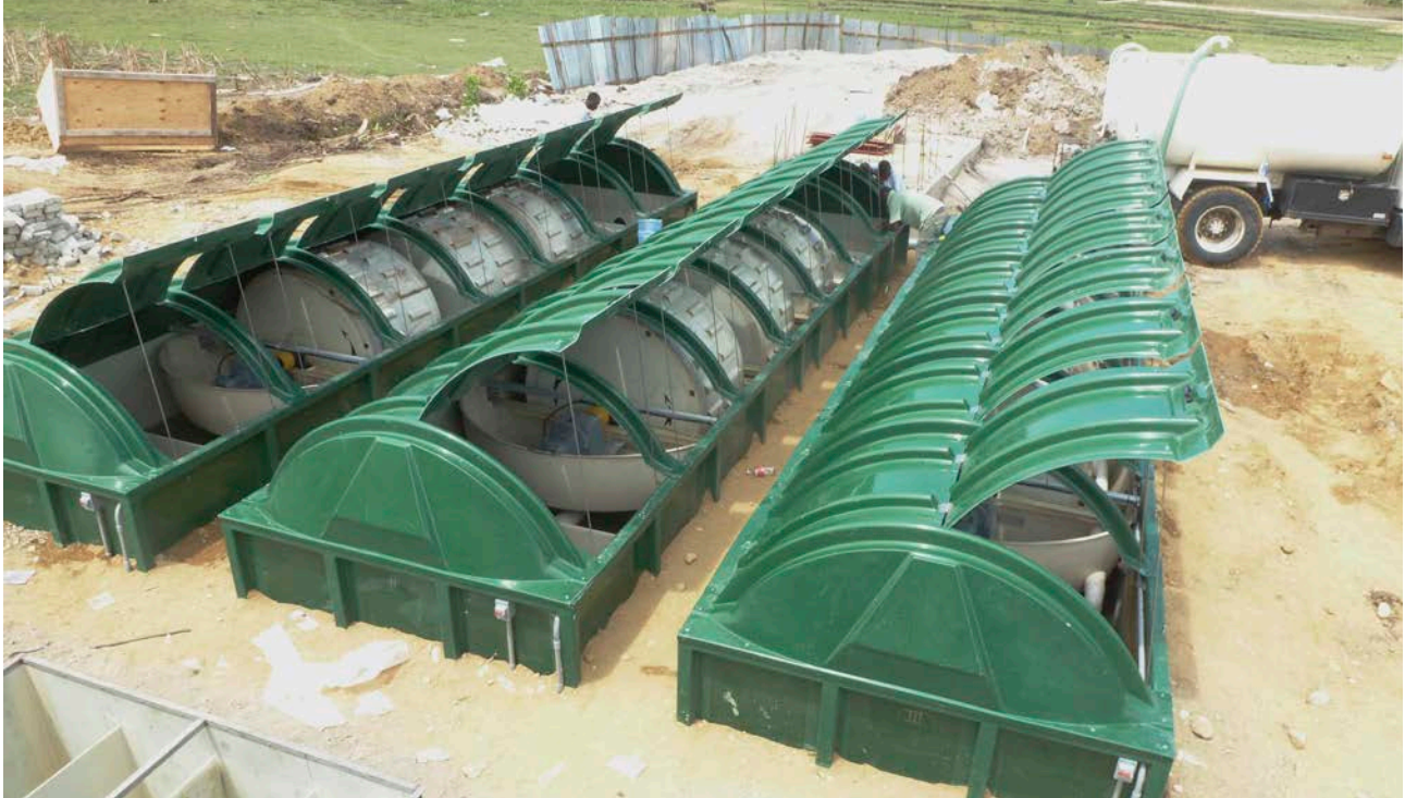
Figure 5.17 Mirebalais Hospital has an on-site modular wastewater treatment system designed for remote applications. The technology achieves aerobic biological treatment by passing the water through several rotating drums. There is solids removal via settling plates at the beginning and end of each unit, with the rotating drums in the middle for biological treatment. The system is compact, efficient in both energy consumption and sludge production, and low-maintenance. Disinfected treated water is discharged to a local tributary of the Artibonite River. Credit: Ann Clark Architects
