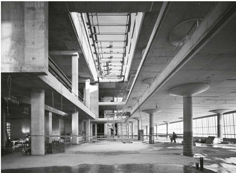
Views of central atrium (top and opposite top); concrete form work during construction (bottom and opposite bottom)
