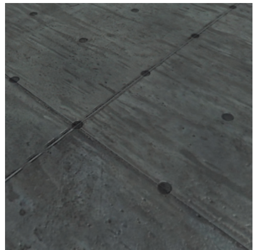
Concrete Formwork Holes
