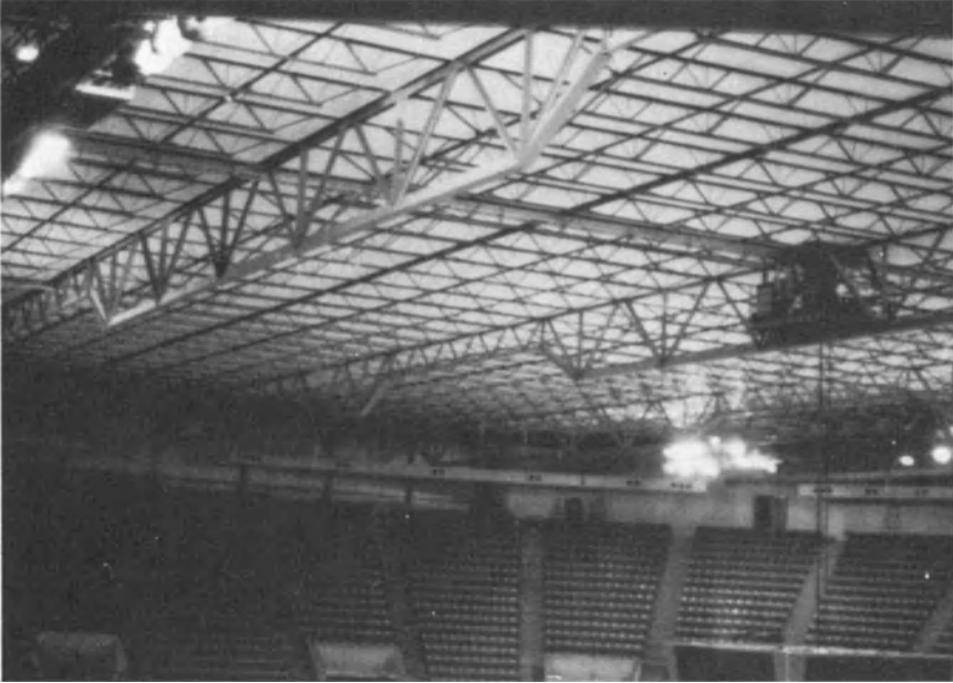
Fig. 3.10. Long-span joist roof system of the American Royal Arena in Kansas City, Missouri (courtesy of U.S. Steel Corp.).
