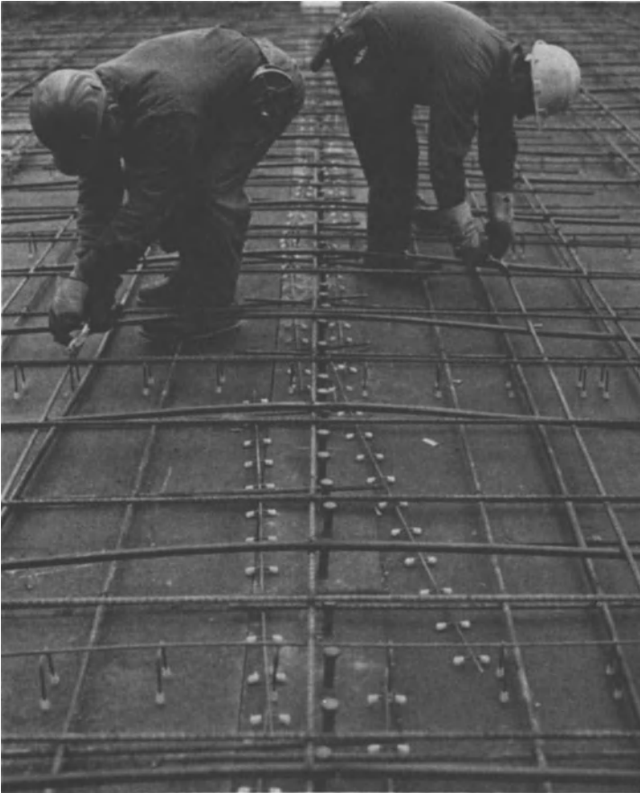
Fig. 9.2. An interior girder of the building whose spandrel beam is shown in Fig. 9.1. Note how reinforcing bars and post-tensioning strands drape over the girder toward the top of the slab to provide negative moment reinforcement.
