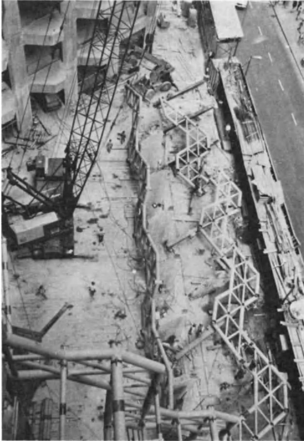
Fig. 0.3. Fabrication of special trusses at a job site to be used for the wall and roof structural system for the atrium lobby of an office building. Note that the trusses, made from tubular sections, are partially prefabricated in the shop to transportable lengths and assembled at the site to form each member.
