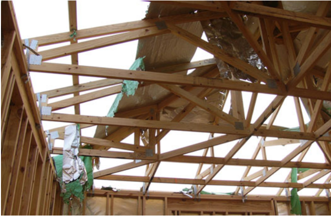
Fig. 4.34 After the storm. Much of the building wrap and roof sarking was removed by strong winds and rain (July 3, 2006)
