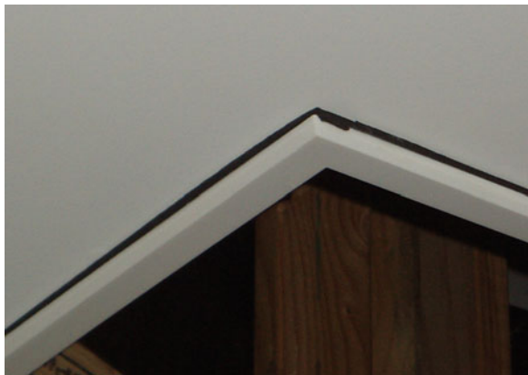
Fig. 4.46 Close up-view of high density foam rubber compressed between prefabricated insert and ceiling (July 21, 2006)
