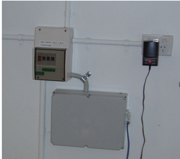
Fig. 4.57 Surface mounted electrical services when finished (August, 2006)
