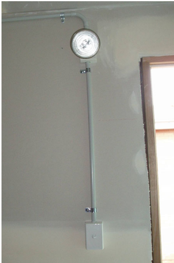
Fig. 4.56 Detail of surface mounted lamp and lamp switch (July 11, 2006)
