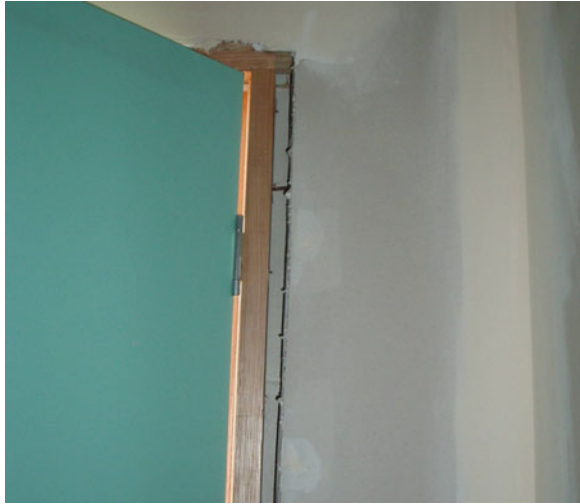
Fig. 4.40 Gap between door jamb and wall frame is clearly visible (July 17, 2006)
