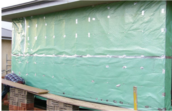
Fig. 4.66 The pattern of silver tape patches shows the location of staples and the effect of insulation installation
