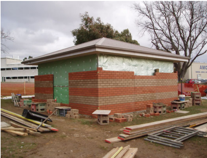
Fig. 4.39 Test cell 3—bricklaying well under way with knock-out panels being left till last (July 10, 2006)
