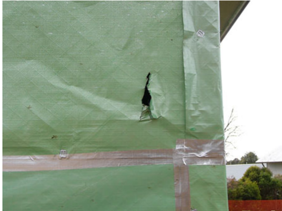
Fig. 4.64 Building wrap torn during construction process
