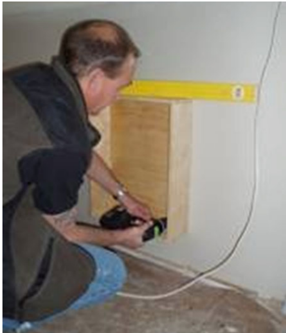
Fig. 4.58 The school technical assistant screw-fixing the heater mounting box to test cell internal wall (July 11, 2006)
