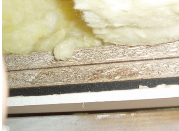
Fig. 4.47 High density foam rubber and particle board sheet affixed to top face of access hatch (July 21, 2006)
