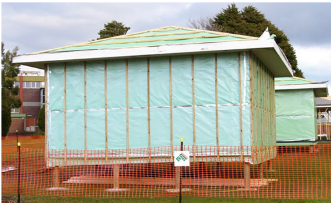
Fig. 4.33 Site photograph at the completion of works on June 30, 2006. Test cell 1 to test cell 3 in receding order
