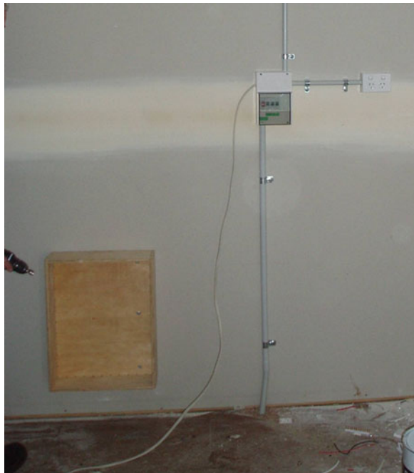
Fig. 4.60 Wall photograph showing proximity of heater to circuit board, and height above floor (July 11, 2006)
