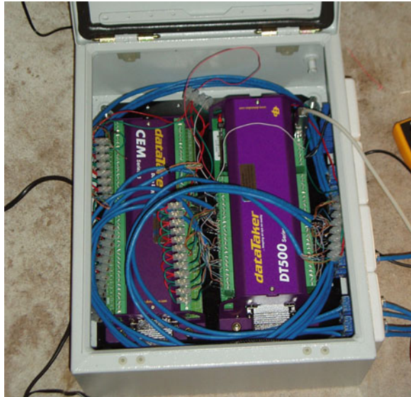
Fig. 4.97 DT500 data loggers and channel expansion module in secure metal case after primary wiring was installed between channels and RJ45 terminals
