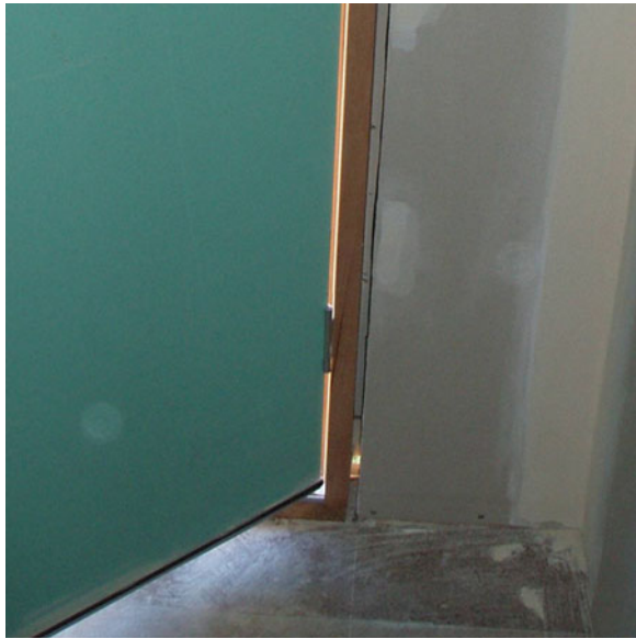
Fig. 4.41 Daylight is visible at the base of the gap between door jamb and wall frame (July 17, 2006)
