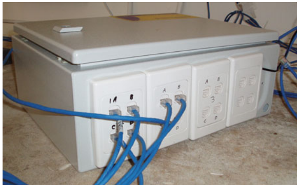
Fig. 4.99 Exterior view of metal data logger box and RJ45 sockets
