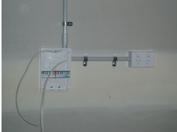
Fig. 4.55 Detail of surface mounted circuit board, conduits and general purpose outlet (July 10, 2006)
