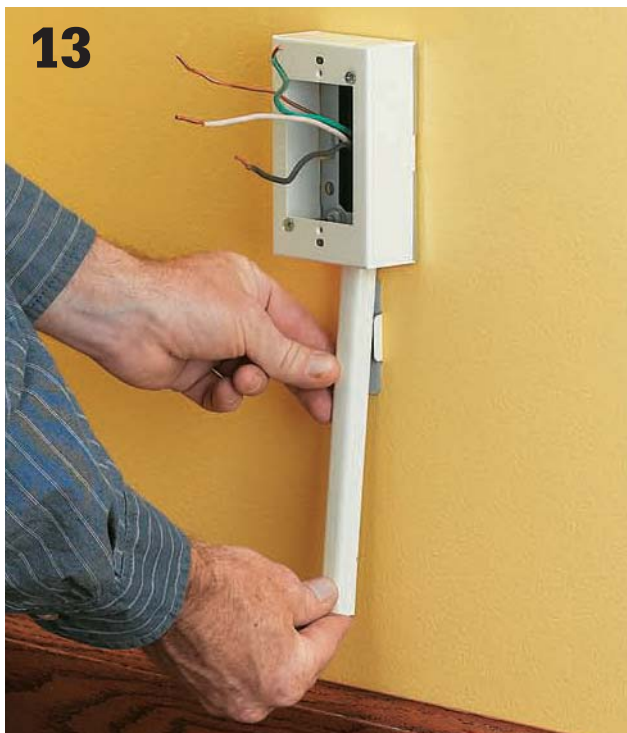
13 At the starter box slide one end of the short piece of raceway into the knockout so that about \frac{1}{8} " extends into the box. Snap the raceway into the clip below the knockout. Repeat this same procedure at the new receptacle box.
