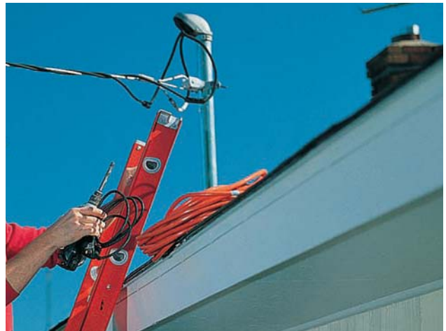
Use fiberglass or wood ladders when making routine household repairs near the service mast.
