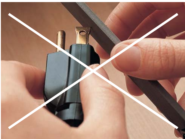
Never alter the prongs of a plug to fit a receptacle. If possible, install a new grounded receptacle.
