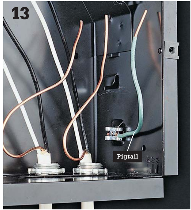
13 At each recessed fixture and metal electrical box, connect one end of a grounding pigtail to the metal frame using a grounding clip attached to the frame (shown above) or a green grounding screw.
