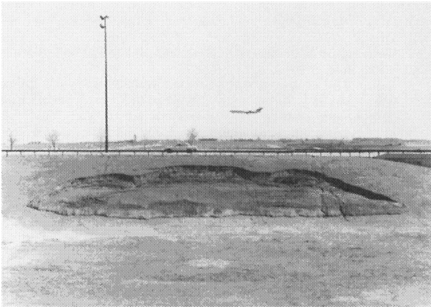
FIGURE 10-1. Typical sliding failure of an earth embankment.
