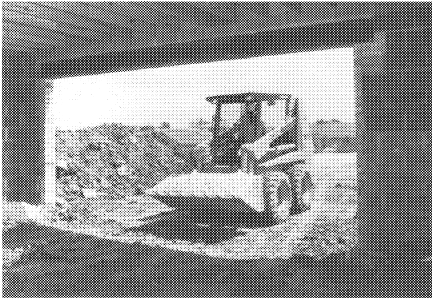
FIGURE D-6. Access as required for the delivery of stone base for use under slab on ground. [Ref. 7]
