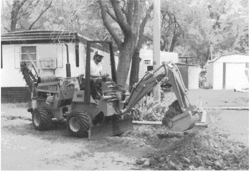
FIGURE 3-3. A backhoe in the process of cutting a trench for visual examination of a soil profile. [Ref. 7]
