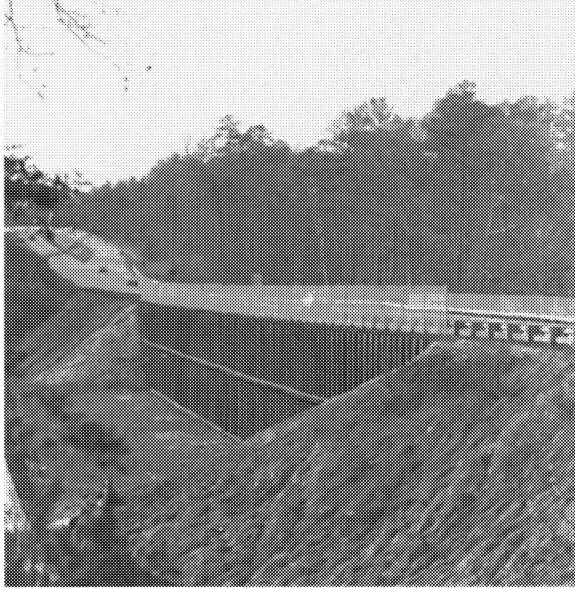
FIGURE 10-4. Bethlehem PZ27 sheet piling stabilizes this busy roadway in a marshy location near Williamsburg, Va. [Ref. 3]
