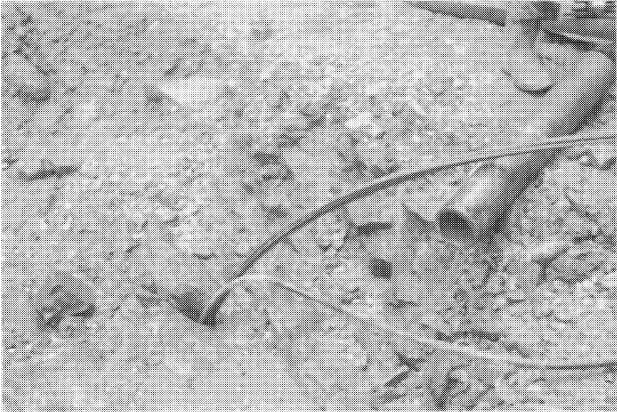
FIGURE 10-23. Rock anchor cable and grout tube positioned in hole prior to grouting the dead end anchorage. [Ref 9]
