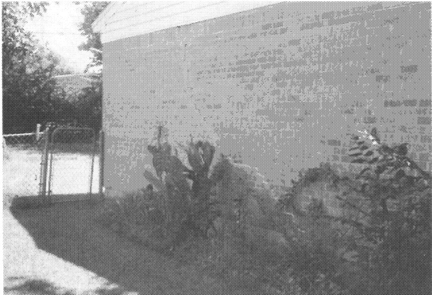
FIGURE 13-7. Damage to a residence, as caused by differential settlement.
