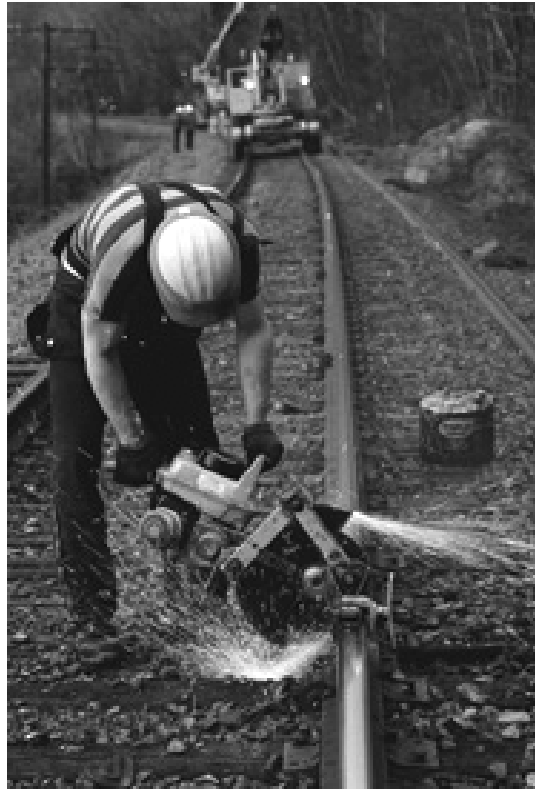
Railway (or "roadway") worker performing repairs on the right-of-way of a railway system
