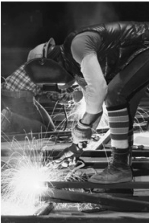
Direct (unprotected) exposure of the eye to a welding arc or other ultraviolet light source is the most common cause of flash burn injuries
