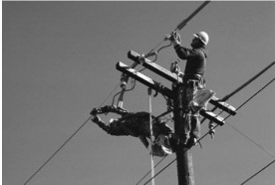
Line workers are exposed to a number of hazards on a daily basis such as working at heights and around high voltage
