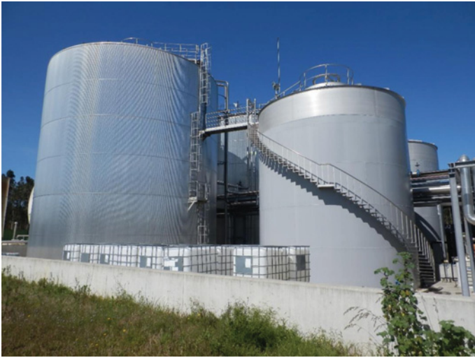
FIGURE 2.20 Single-stage continuous anaerobic digesters (at the left is the digester, at the right is the suspension buffer tank). Courtesy: Valorlis, S.A.
