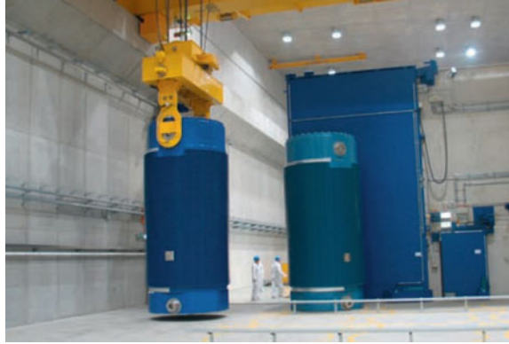
Fig. 7.3 Intermediate storage facility (dry storage) with CASTOR casks [7]
