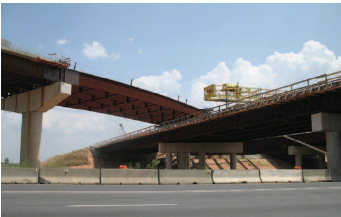
Figure 3.1 Construction of the outerbelt freeway around Charlotte, NC. This 60-mile circular freeway around the city has taken more than 10 years to build and cost more than a billion (US) dollars.
