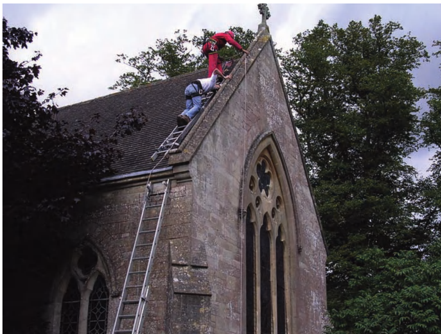
Figure 16.2 Inspection of high-level areas raises health and safety issues. One response is to use roped access, as on this Gloucestershire church.
