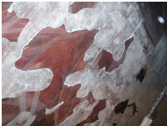
Fig. 3.3 Image of a portion (area ca. 1 \text{ m}^2 ) of the damaged Palomino's frescoes in the vault of the Sant Joan del Mercat church in Valencia (Spain) [133]
