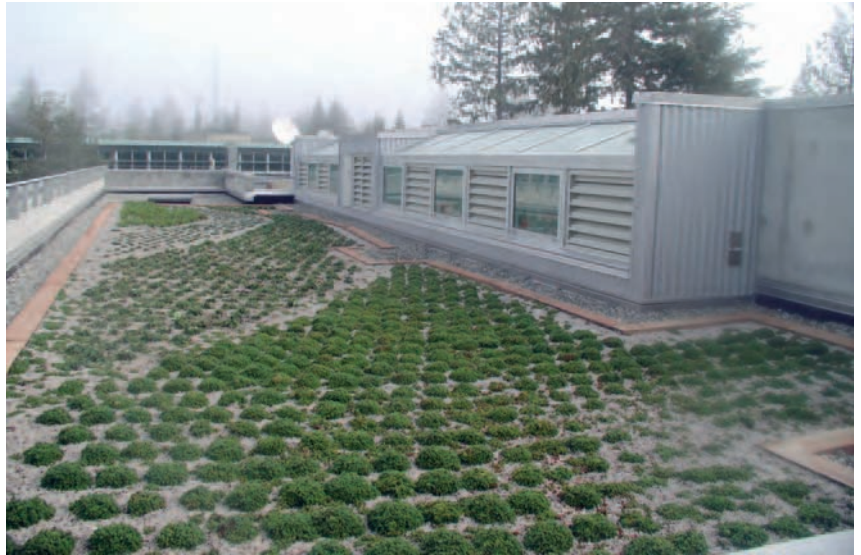
► 7.1 The Evergreen State College campus expansion project features a green roof on the LEED-NC Gold-certified project. Courtesy of DPR Construction.
