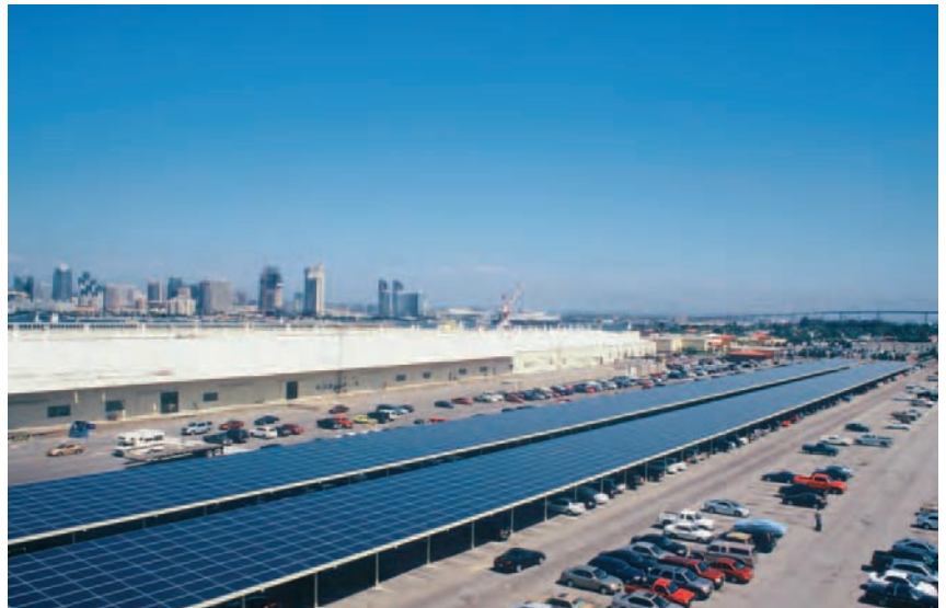
► 7.3 The 924-kilowatt PV system installed by PowerLight on the carport at the US Naval Base in Coronado, California generates enough energy during the day to power over 935 homes. Courtesy of SunPower Corporation.
