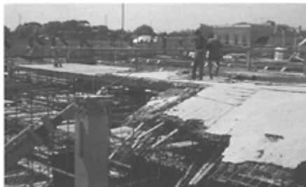
Result of Progressive Formwork Collapse
