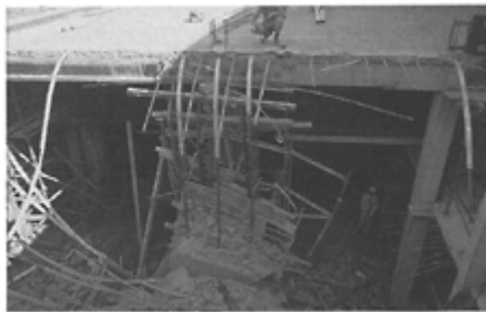
A Formwork Failure
