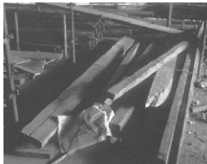
Damaged Formwork Materials
