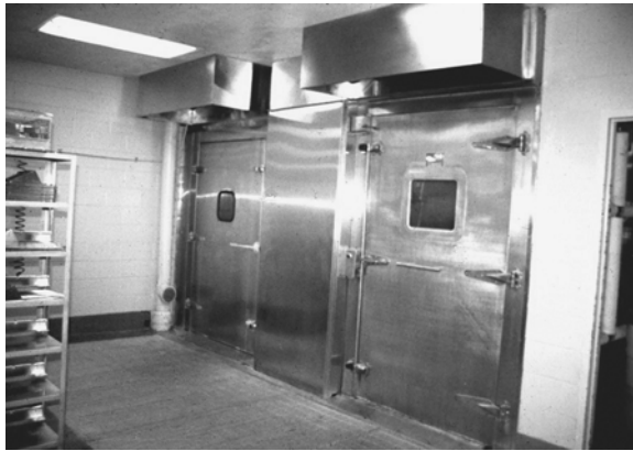
Figure 8.20 A view of a pair of batch-type cage and rack washers from the clean side of the cage sanitation area that are pit mounted to make the washer floor level with the room floor. Note the exhaust fume hoods at the ceiling and the grate-covered pit in front of the washers.
