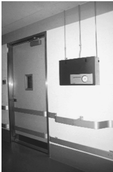
Figure 8.15 A corridor in an animal facility showing extruded solid aluminum bumper guardrails at two levels to protect the walls and the door. If only one guardrail is to be used, the lower one may provide the most protection from the widest variety of mobile equipment. Note that the rail extends further out from the wall in one location to protect wall-mounted equipment that protrudes further from the wall than the typical rail mounting of 3 in from the wall.
