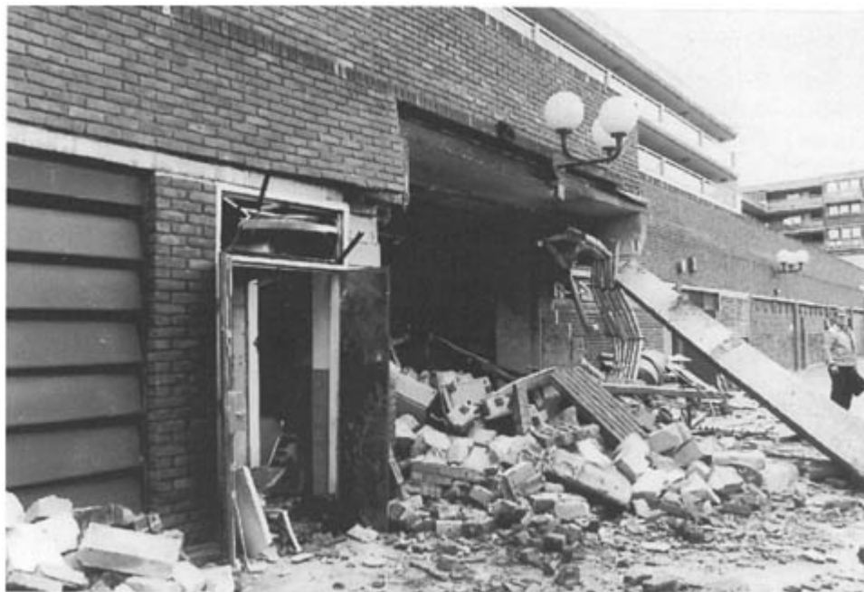
Figure 7.8 Structural damage caused by a bursting electrically heated hot water cylinder.
