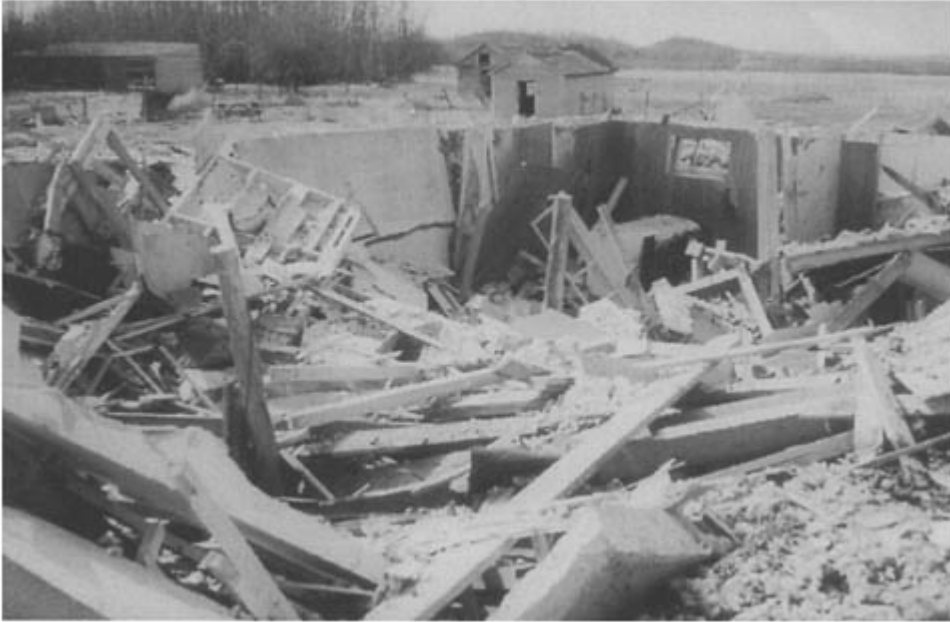
Figure 4.6 The aftermath of a natural gas explosion—the basement.
