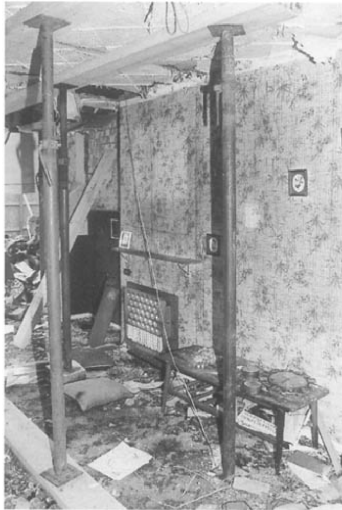
Figure 7.27 View of lounge showing scorched wallpaper, coffee table and carpet, and the 'Baxi' boiler.
