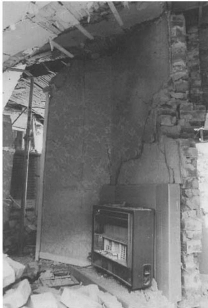
Figure 7.10 Thermal damage to a wall caused by deflagration of a natural gas/air mixture.
