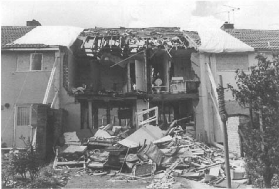
Figure 7.26 Rear view of the damaged building (dwelling B).
