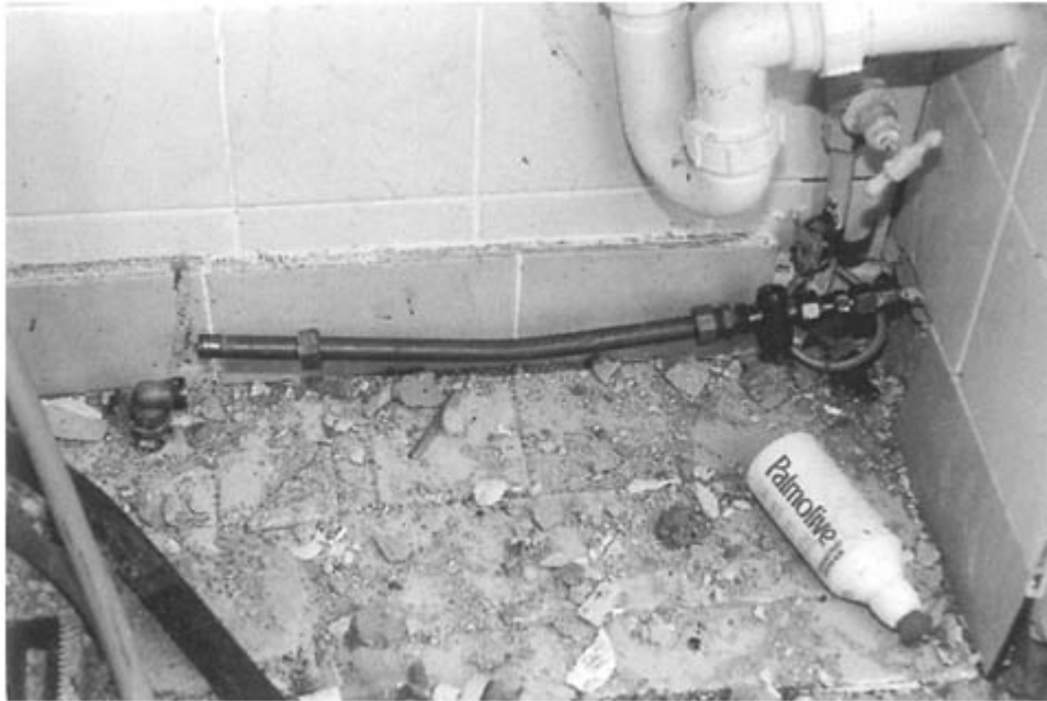
Figure 7.28 The failed compression fitting.
