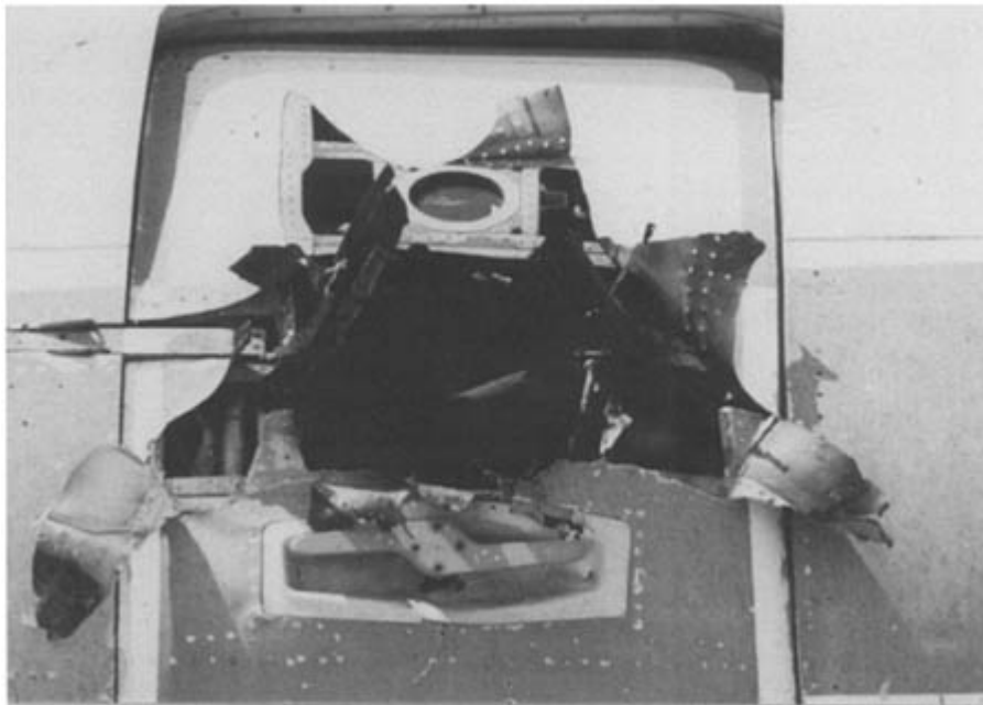
Figure 6.15 Side view of an irregular-shaped radial burst pattern in the exterior skin of a transport aircraft following the detonation of a small improvised explosive device.
