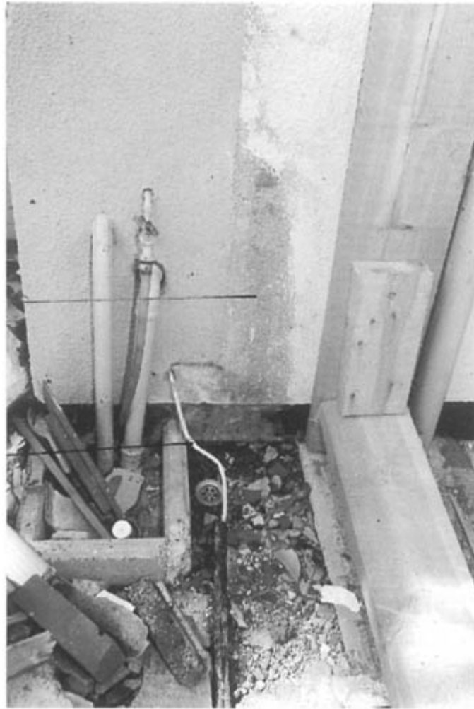
Figure 7.29 Basic 9 mm sleeved pipe emerging from the external wall of the kitchen.
