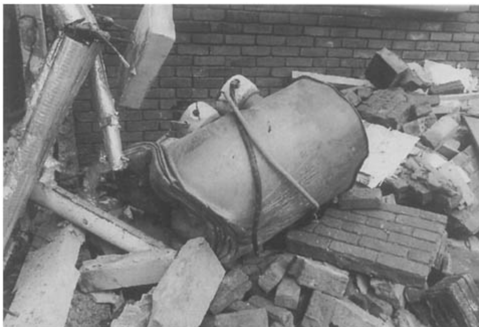
Figure 7.9 Electrically heated hot water cylinder, which had burst.
