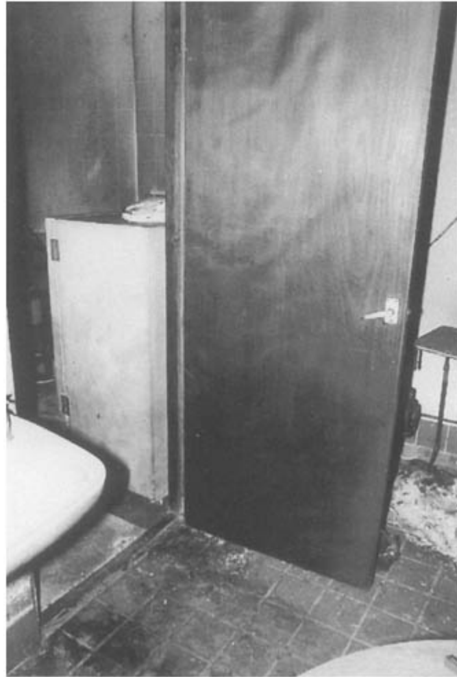
Figure 7.12 Scorching to the bottom of a door and refrigerator caused by deflagration of a gasoline/air mixture.
