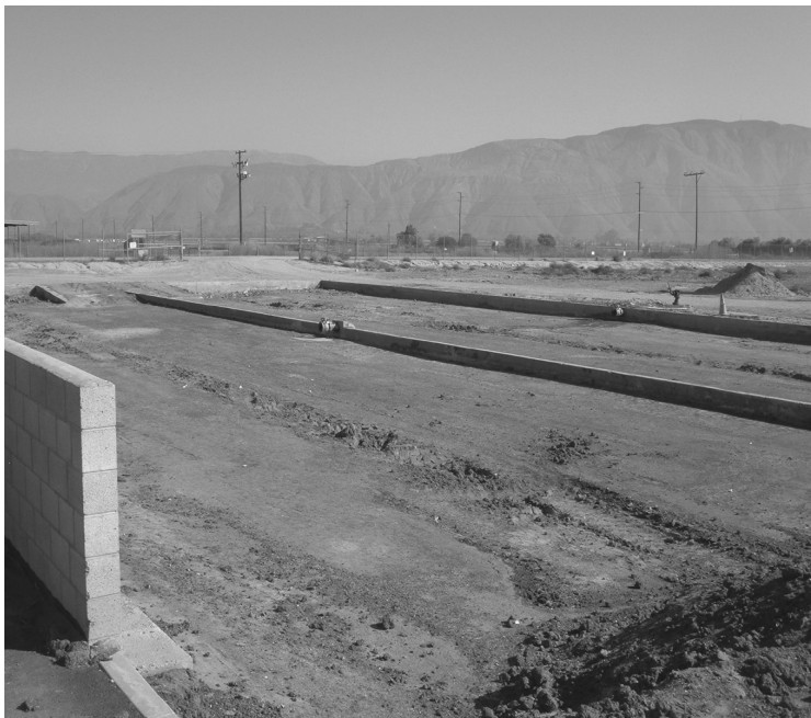
Figure 5.5.39a View of Sand Drying Beds
