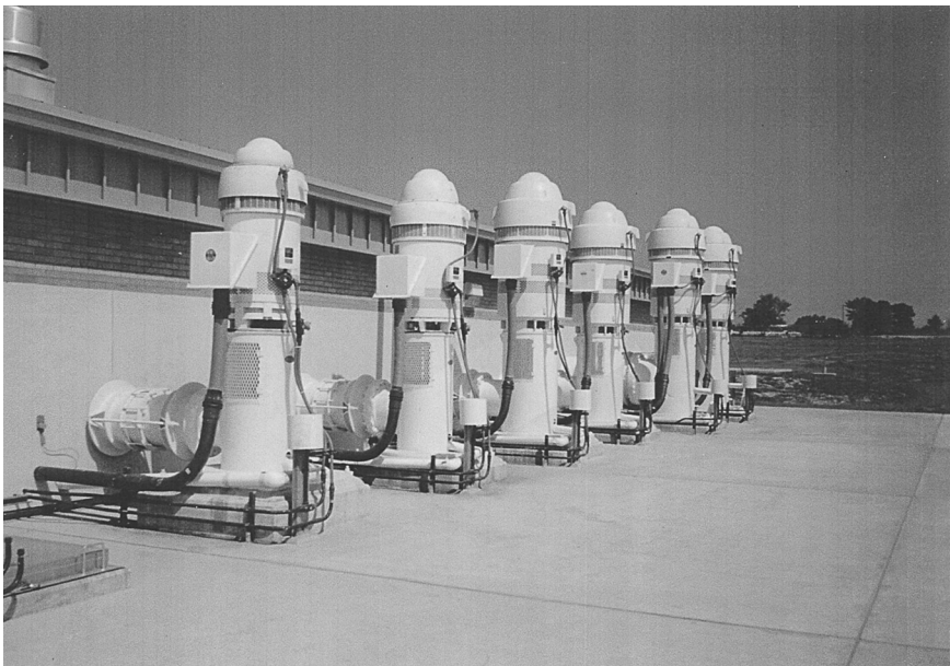
Figure 5.5.36a Six Vertical Pumps in Front of a Building
