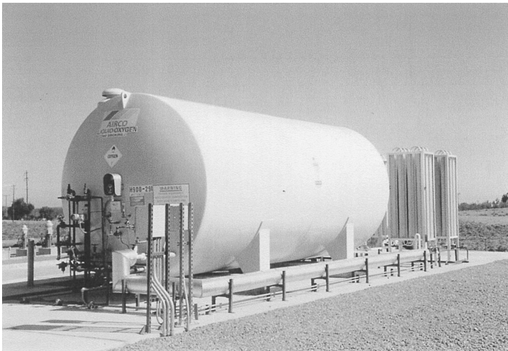
Figure 5.5.4b Liquid Oxygen Storage Tank and Evaporators
