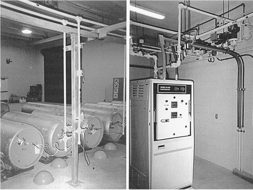
Figure 5.5.1a One-Ton Chlorine Cylinders and Chlorine Feeder
