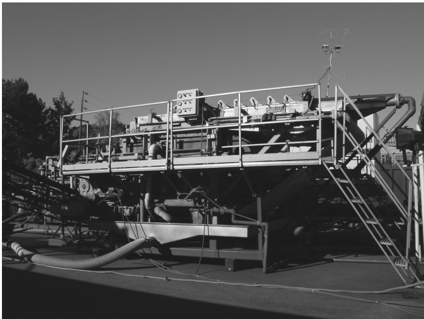
Figure 5.5.41a View of Filter Belt Press
