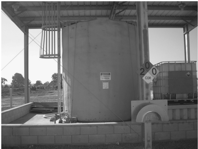
Figure 5.5.7a Alum-Polymer Storage Tank
