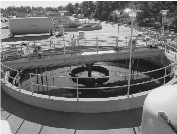
Figure 5.5.37a Gravity Sludge Thickener
