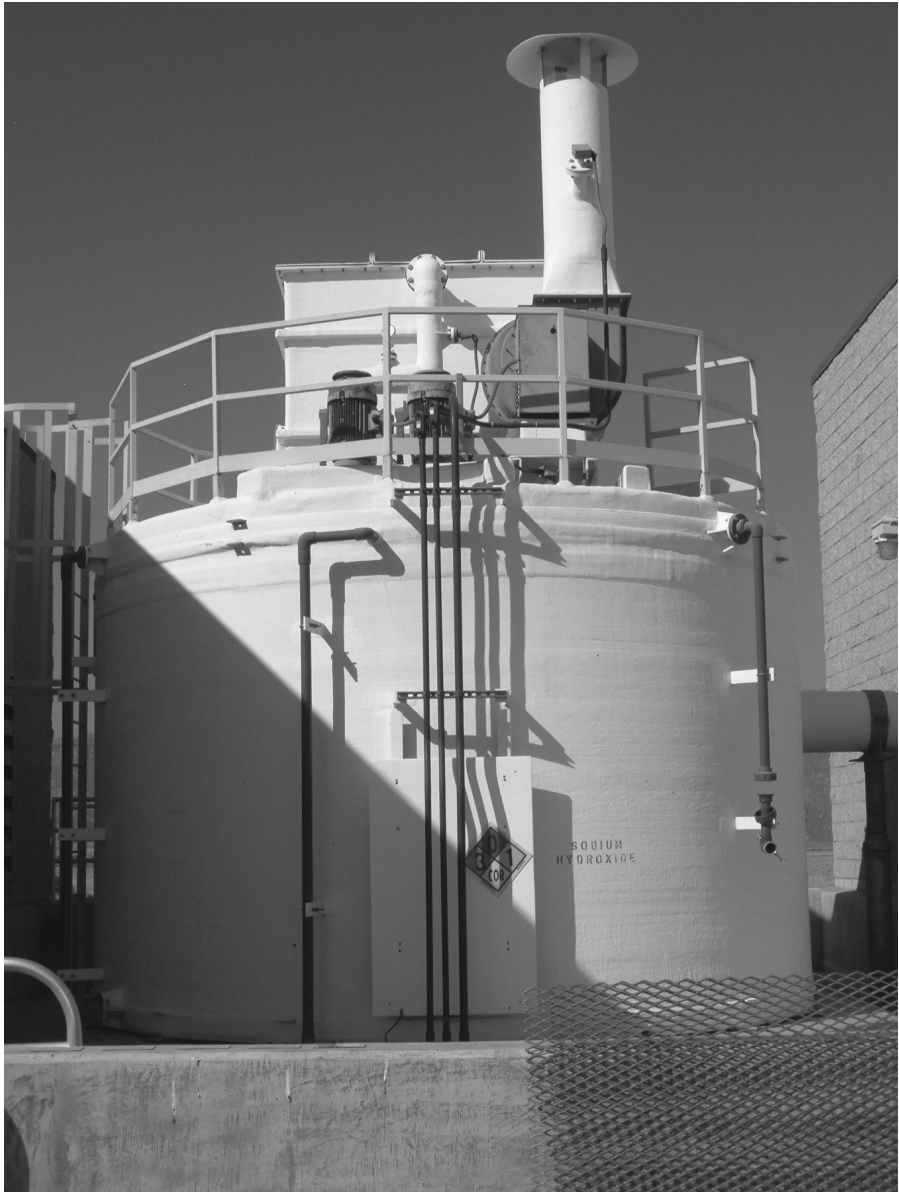
Figure 5.5.12a Sodium Hydroxide Storage
