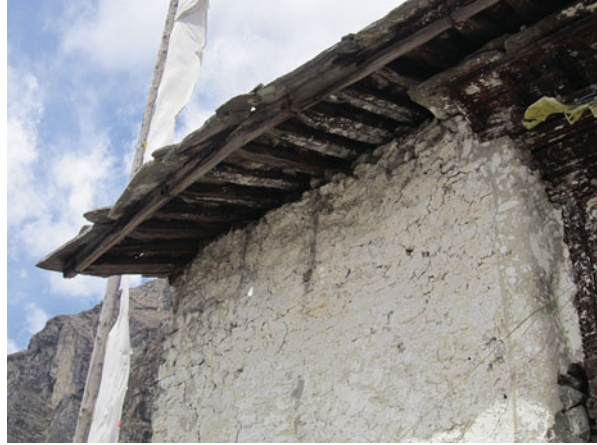
Fig. 3.4 The open joist arrangement of the Langtang gompa (photographs by Hayley Saul)
