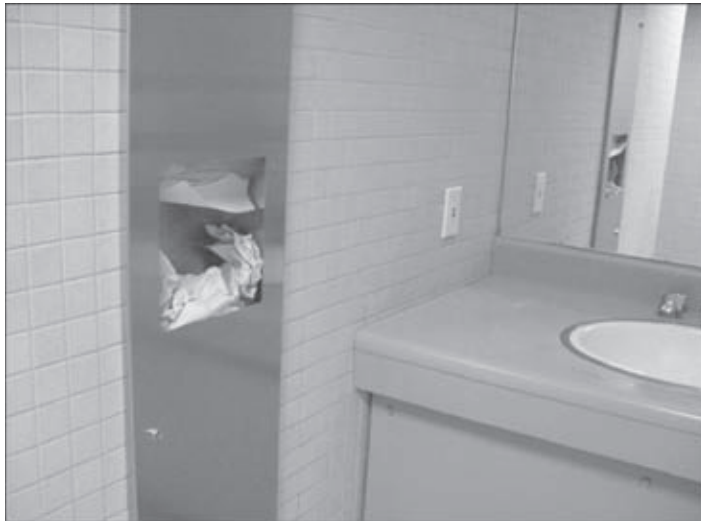
PHOTO 3.1. Poorly Designed Paper Towel Dispenser and Disposal Unit.
