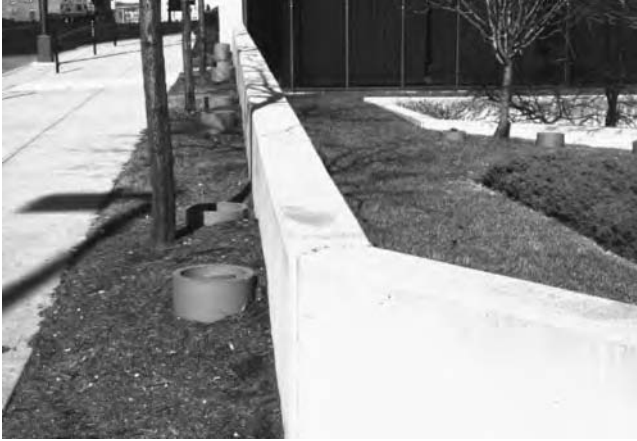
Figure 13.7 Narrow tree planting zones pre-dispose the design to pavement damage if the trees are successful in surviving and growing. (Photo credit: E. Gilman.)
