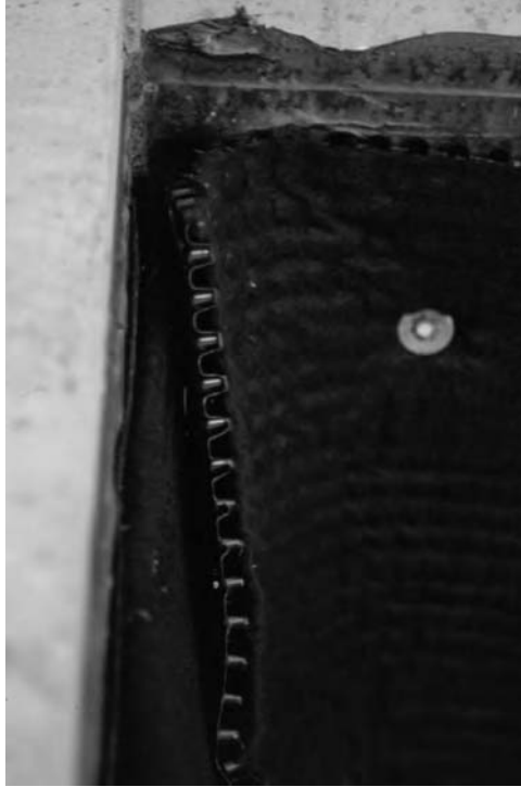
Figure 13.21 Interior drainage geocomposite for a sealed container positioned on the sides of the container. (Photo credit: E. Gilman.)
