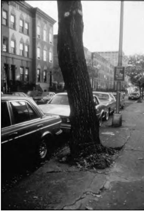
Figure 13.9 Trees and pavement grow older together, but as the tree grows, the concrete simply ages. Time, traffic, and the soil materials under the sidewalk influence the damages caused by root growth under the pavement. (Photo credit: N. Bassuk.)
