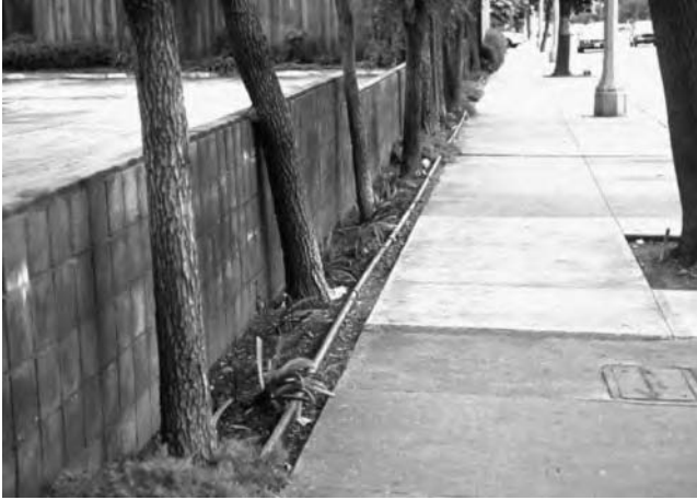
Figure 13.5 The width of a berm or any other root zone must factor in the width of a minimal root plate for stability and avoidance of root-pavement problems: A fact lost on the author of this planting design. (Photo credit: E. Gilman.)
