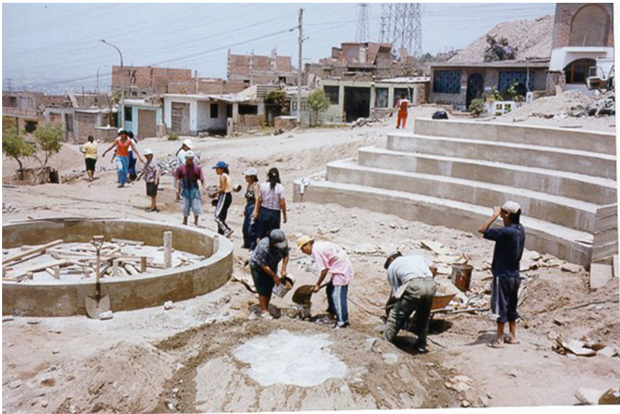
Fig. 2 The construction of the amphitheater by the residents of 20 de Mayo in 2000 (Source: Veronica Rondon Rodriguez took this picture in 2000)
