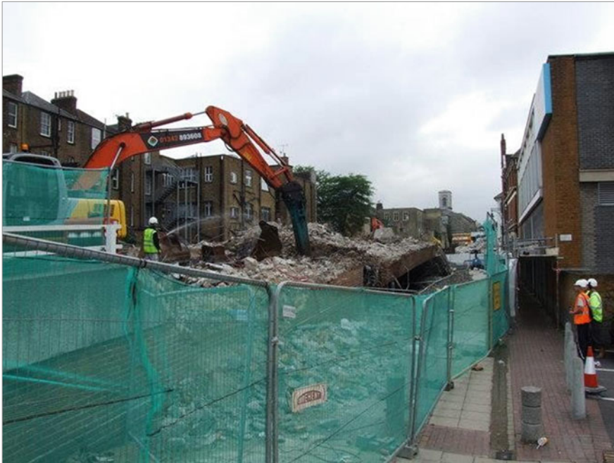
Fig. 6.3 Flyover Demolition, Chatham, UK. Source Photograph by Chris Whippet. Licensed under CC BY-SA 2.0 via Wikimedia Commons; Flyover Demolition at Chatham U.K https://commons.wikimedia.org/wiki/File:Flyover_Demolition,_Chatham_-_geograph.org.uk_-_1437084.jpg#/media/File:Flyover_Demolition,_Chatham_-_geograph.org.uk_-_1437084.jpg
