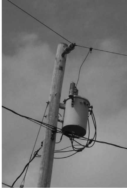
FIGURE 11.9 Single-phase overhead distribution transformer.
