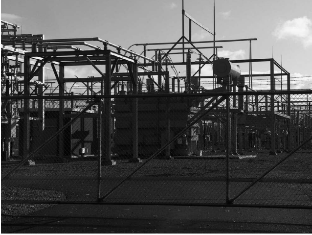
FIGURE 11.1 Representative substation with overhead bus and substation transformer.
