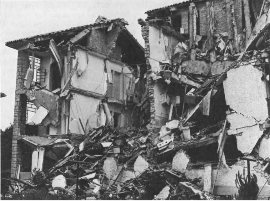
Figure 6.5. Gemona del Friuli, Italy: View of Damaged Buildings after Earthquake of May 6, 1976.
