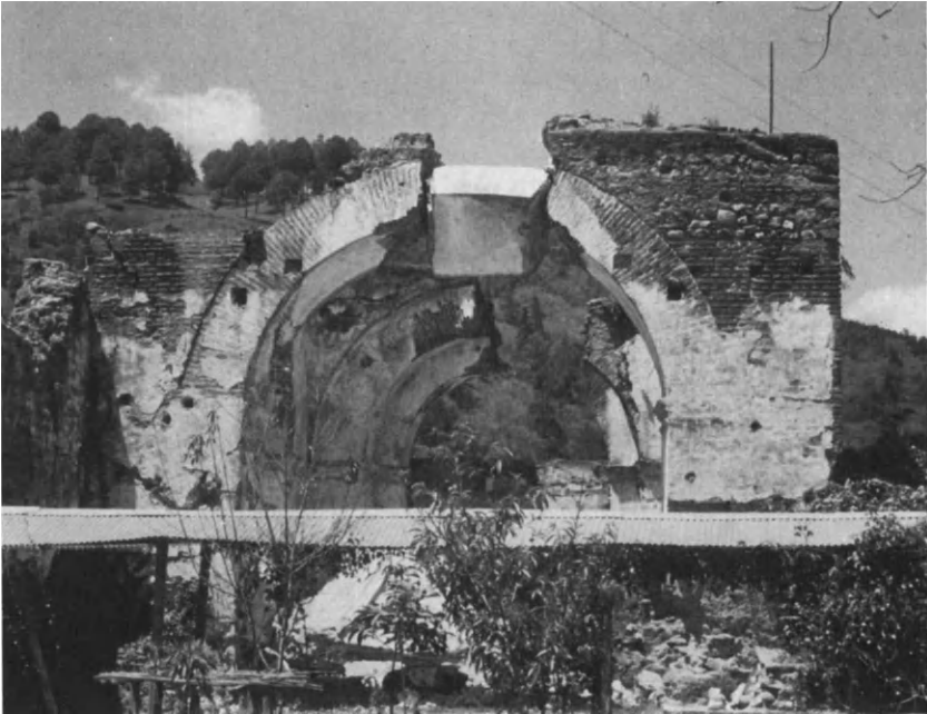
Figure 5.15. Antigua Guatemala, Guatemala: Church of San Francisco, Transept Arch Showing Dislodged Central Portion after Earthquake of February 4, 1976.
