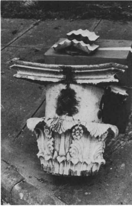
Figure 5.36. Montgomery, Alabama: Alabama State Capitol, 1850, Deteriorated Wooden Capital.
