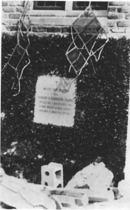
Figure 5.30. Mobile, Alabama: Trinity Episcopal Church, Henry Dudley and Frank Wills, Archs., 1853, Damage to Leaded Glass from Hurricane Frederick, September 12-13, 1979.
