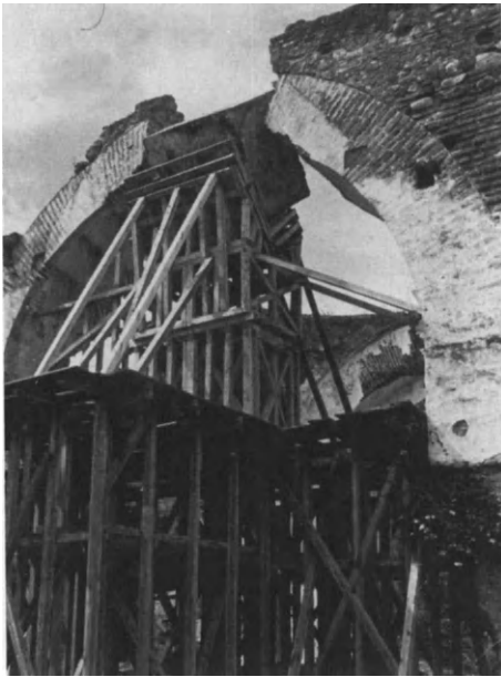
Figure 5.16. Antigua Guatemala, Guatemala: Church of San Francisco, Transept Arch Showing Platform Designed to Support Central Portion.
