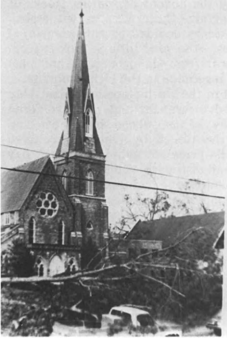
Figure 5.20. Mobile, Alabama: Trinity Episcopal Church, Henry Dudley and Frank Wills, Archts., 1853, Damage from Hurricane Frederick, September 12, 1979.
