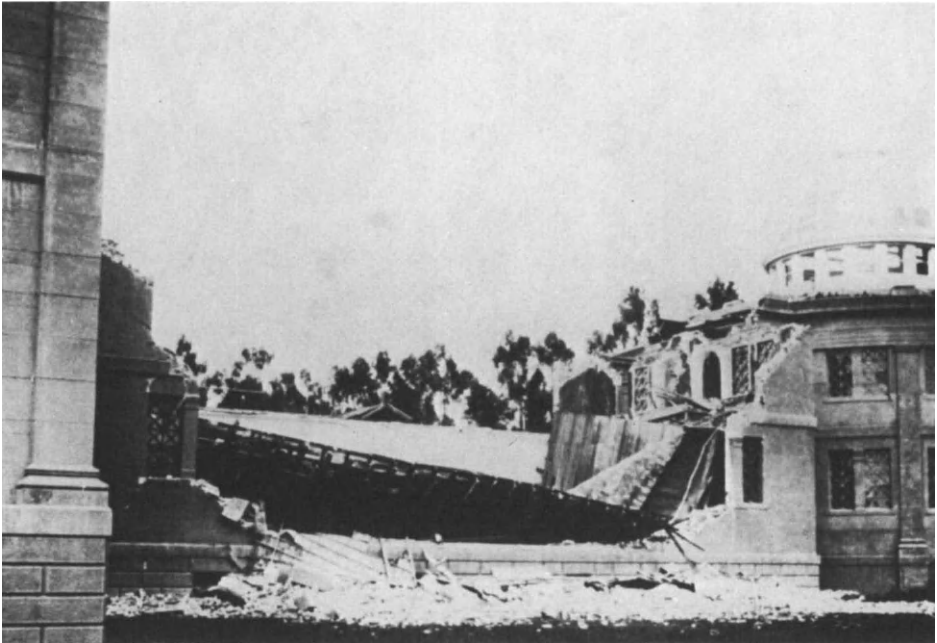
Figure 3.4. Palo Alto, California: Stanford University Museum, Shepley, Rutan and Coolidge, Archs., 1887-1891, Damage from Earthquake of April 18, 1906. USGS.
