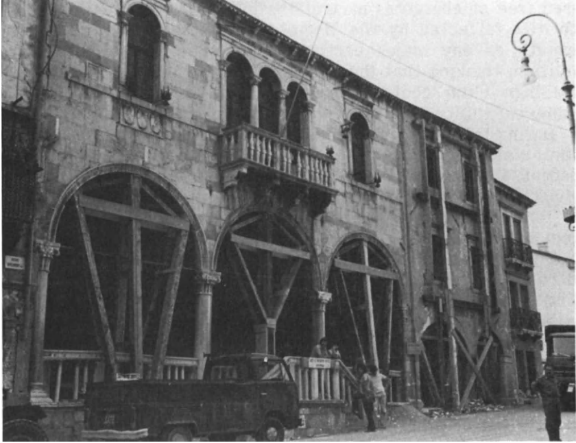
Figure 5.3. Gemona del Friuli, Italy: Palazzo Comunale, Built in 1502, Showing Bracing Erected After Earthquake of May 6, 1976.
