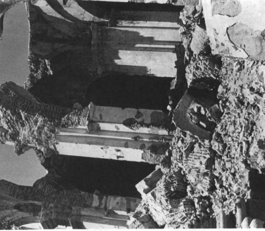
Figure 5.10. Antigua Guatemala, Guatemala: Cathedral, Side Aisle Elliptical Vault Showing Destruction Caused by Battering of Concrete Ribs in Earthquake of February 4, 1976.
