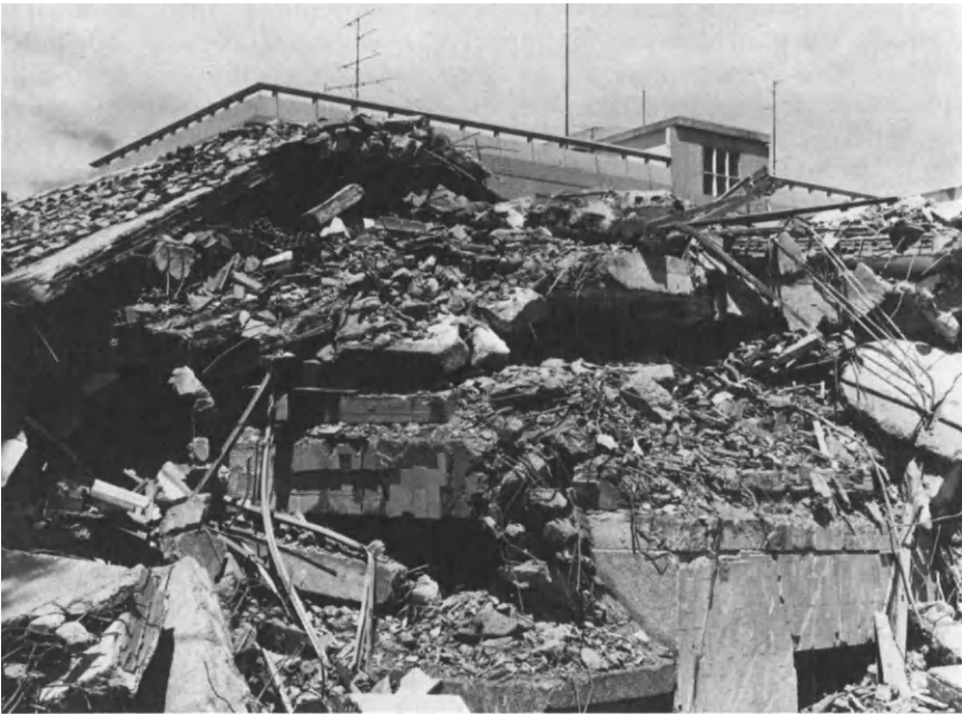
Figure 6.6. Gemona del Friuli, Italy: View of Pancaked Modern Reinforced Concrete Structure after Earthquake of May 6, 1976.
