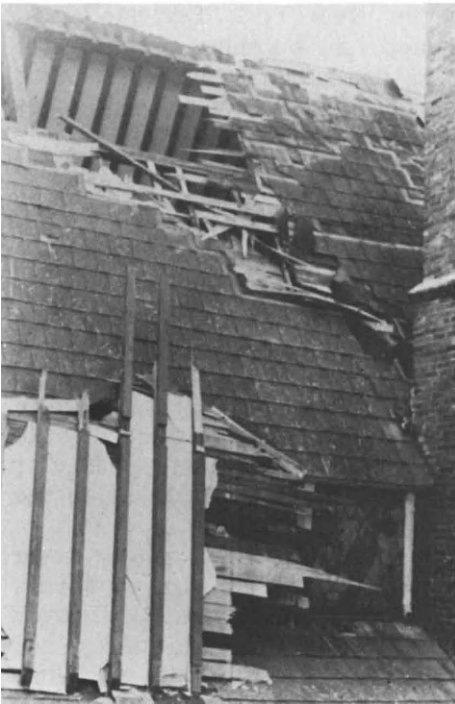
Figure 5.21. Mobile, Alabama: Trinity Episcopal Church, Henry Dudley and Frank Wills, Archts., 1853, Damage to Roof of Nave from Hurricane Frederick, September 12, 1979.
