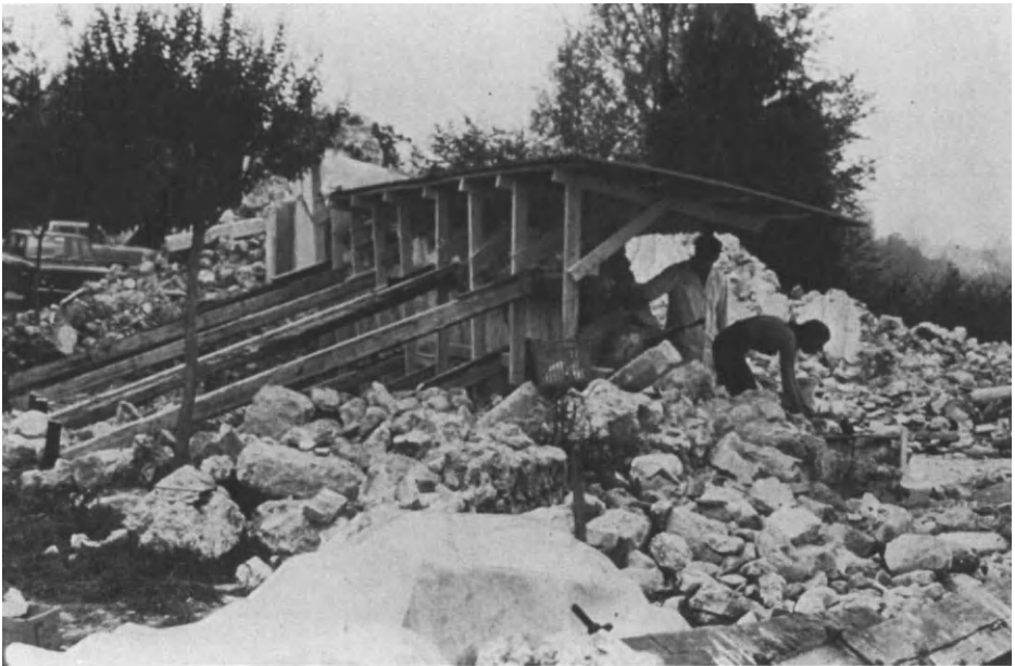
Figure 1.25. Villuzza of Ragogna, Italy: Church of San Lorenzo, Propping and Temporary Roofing Constructed to Protect Frescoes on Walls Which Were to Remain in situ.
