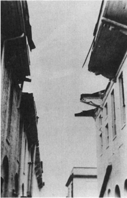
Figure 5.32. Mobile, Alabama: Damage to Eaves of Houses by Hurricane Frederick, September 12, 1979.
