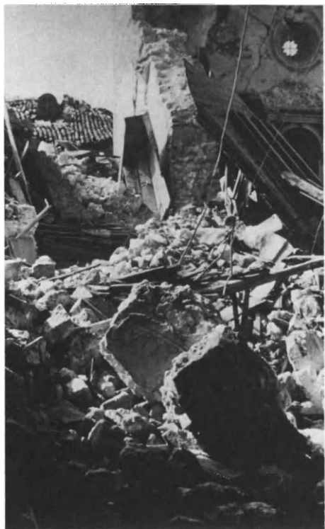
Figure 1.19. Gemona del Friuli, Italy: Church after Earthquake of May 6, 1976.
