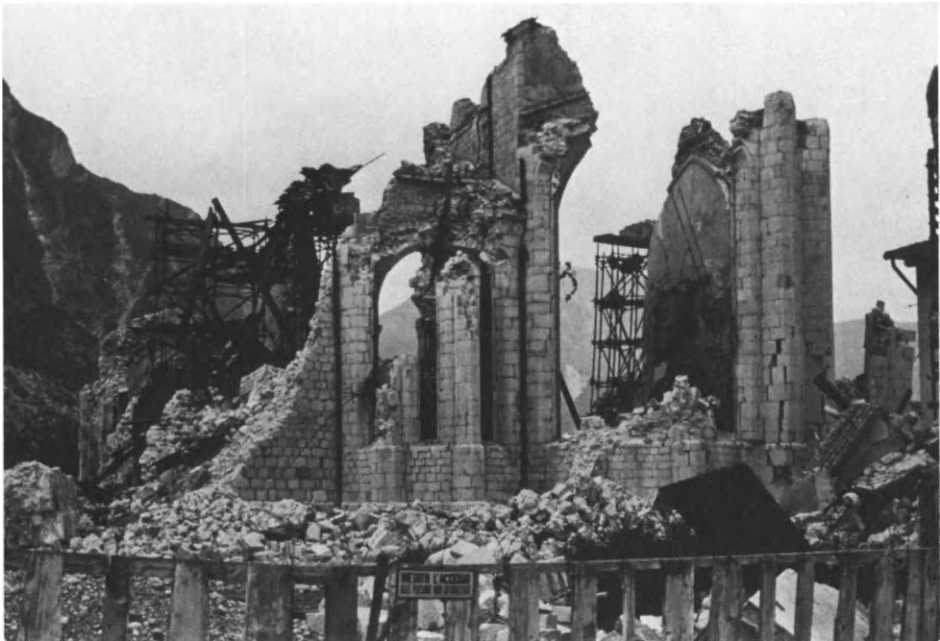
Figure 1.27. Venzone, Italy: Cathedral after its Collapse in Earthquake of September 15, 1976.
