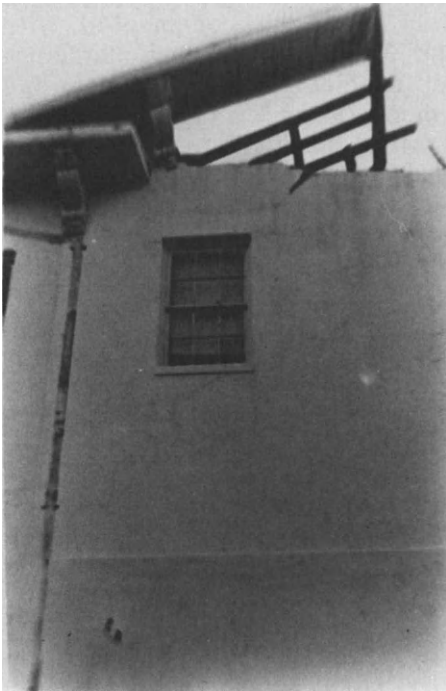
Figure 5.41. Mobile, Alabama: Mobile City Hall, 1854, Gable Wall Blown into Attic by Hurricane Frederick, September 12, 1979.
