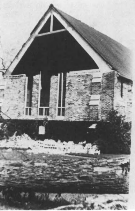
Figure 5.22. Mobile, Alabama: Trinity Episcopal Church Parish House, 1960's, Showing South Wall which Fell Outward Through Suction during Hurricane Frederick, September 12, 1979.
