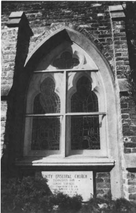
Figure 5.31. Mobile, Alabama: Trinity Episcopal Church, Henry Dudley and Frank Wills, Archs., 1853, Leaded Glass Protected by Lexan after Hurricane Frederick, September 12-13, 1979.
