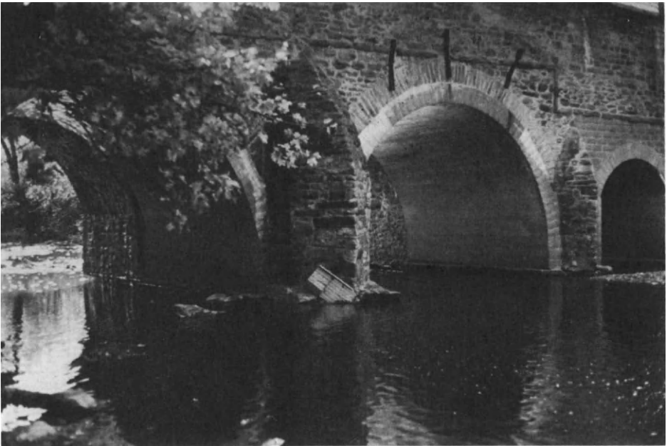
Figure 3.26. Philadelphia, Pennsylvania: Frankford Avenue Bridge over Pennypacker Creek Built in 1694 Showing Metal Straps Reinforcing Center Arch.
