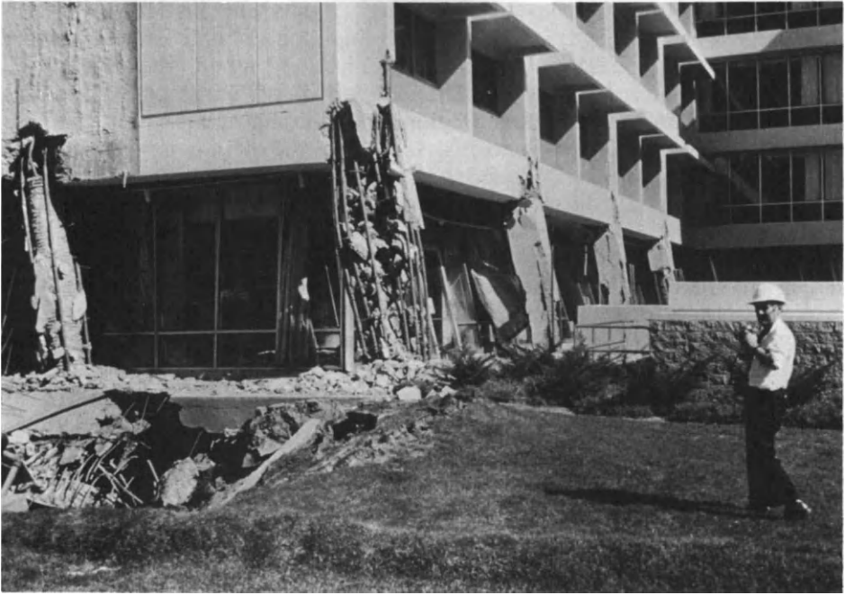
Figure 3.47. Sylmar, California: Olive View Hospital Showing Damage from San Fernando Earthquake of February 9, 1971.
