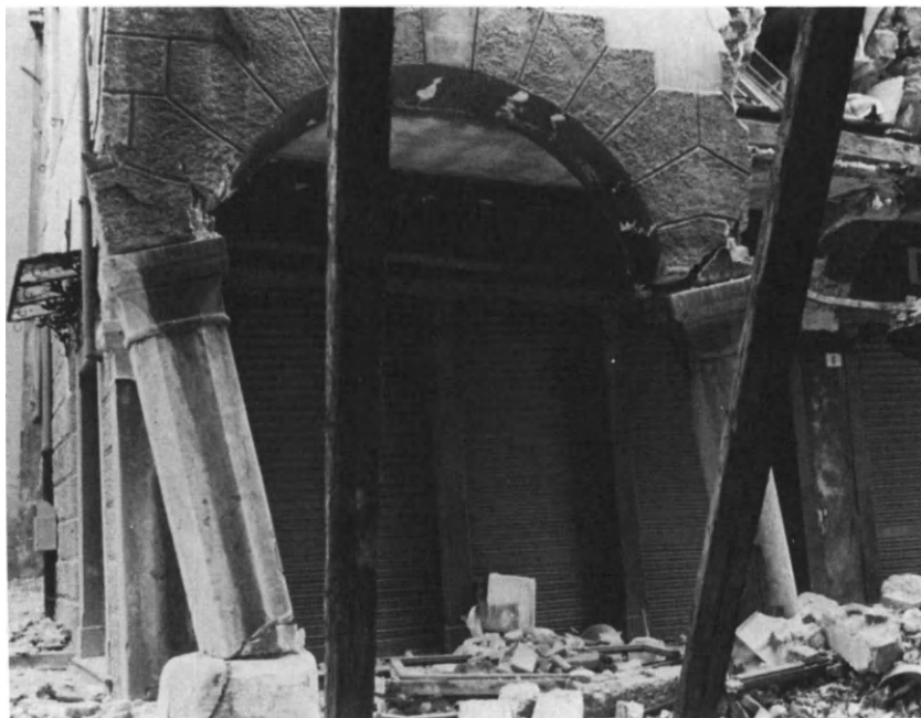
Figure 5.1. Gemona del Friuli, Italy: Ground Story of Dwellings on the Main Street after Earthquake of May 6, 1976.
