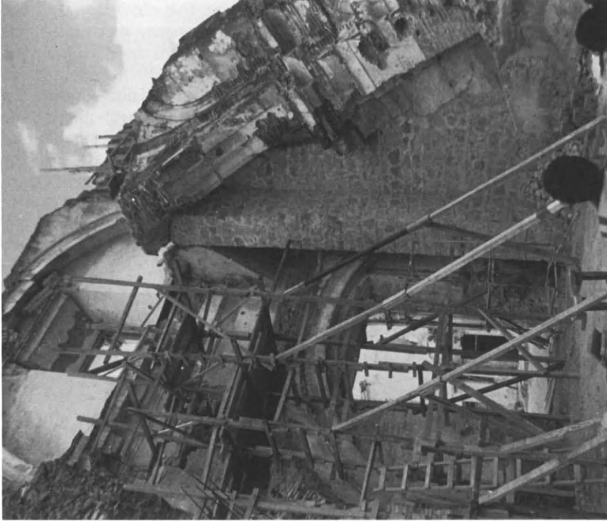
Figure 5.14. Antigua Guatemala, Guatemala: Compañía de Jesús, Main Facade Showing Removal of Concrete Connectors and Separate Buttrressing of Rear of Facade and Leaning Pillar of Nave.
