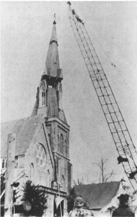
Figure 5.23. Mobile, Alabama: Trinity Episcopal Church, Henry Dudley and Frank Wills, Archts., 1853, Removal by Sections of Steeple Damaged by Hurricane Frederick, September 12, 1979.
