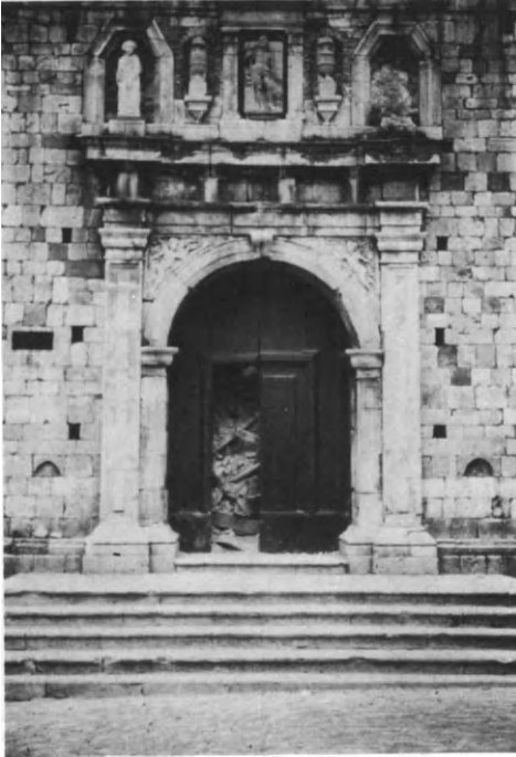
Figure 1.15. Campania-Basilicata, Italy: Church Facade after Earthquake of November 23, 1980.
