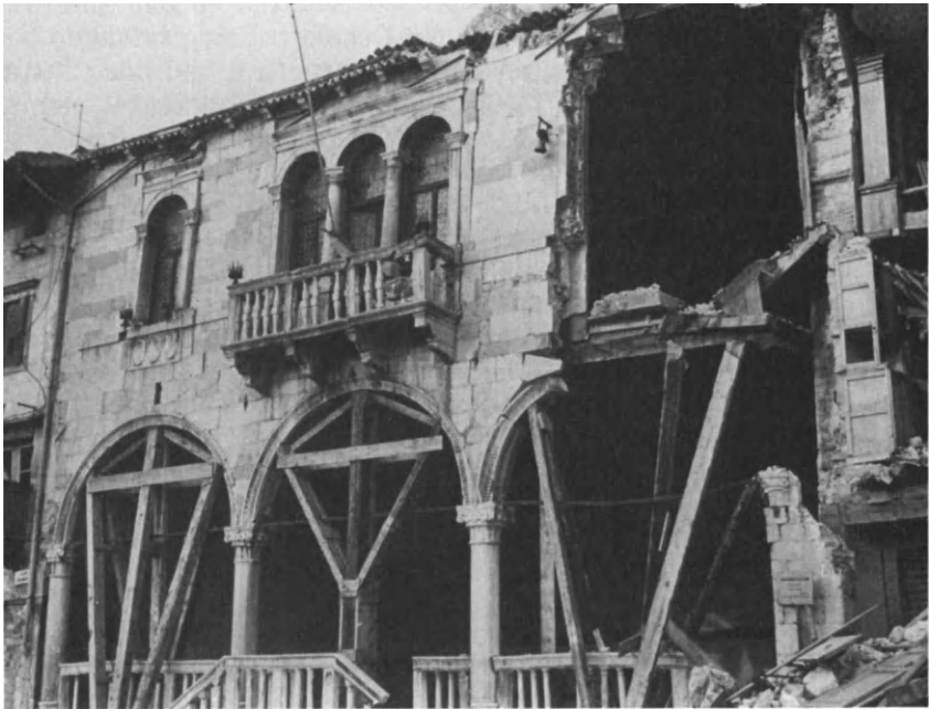
Figure 5.4. Gemona del Friuli, Italy: Palazzo Comunale, Built in 1502, Showing Destruction Following Earthquake of September 15, 1976.
