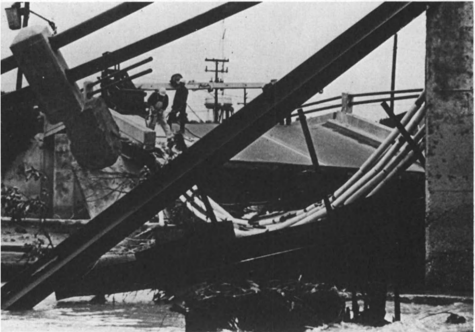
Figure 3.21. Arlington, Virginia: Flood Damage to Bridge Following Hurricane Agnes, June 22, 1972.
