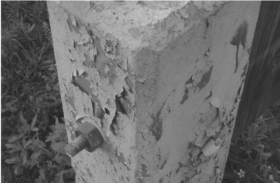
A real-world example of old peeling paint on a concrete barricade post
