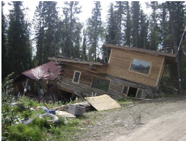
FIGURE 6-1 Eagle, Alaska, July 27, 2009. Don and Judy Mann's house in Eagle, Alaska, was pushed 300 feet off its foundation by ice and floodwaters this past spring. They are rebuilding through the assistance of FEMA and volunteers.
