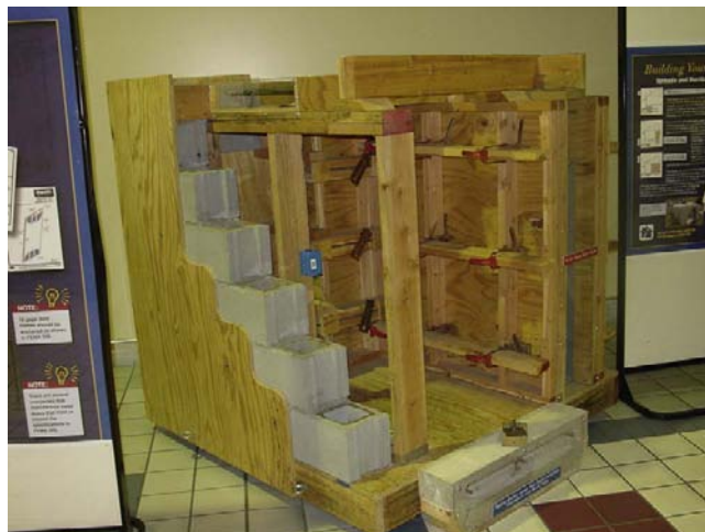
FIGURE 2-4 Tulsa, Oklahoma, November 23, 2001. Disaster Ally in the Eastland Mall. Safe rooms can be designed with many different materials. Shown are concrete block walls, formed concrete walls, and a special ceiling framing. Photo by Kent Baxter/FEMA News Photo.
