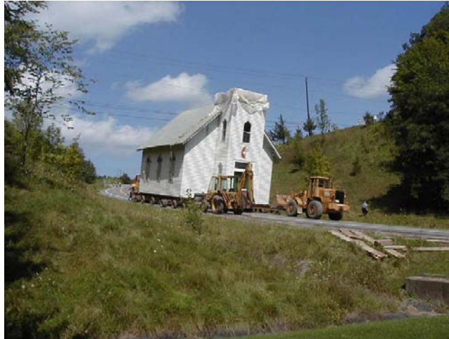
FIGURE 3-6 Albany, New York. This church is being moved half a mile to higher ground as part of the Stryker Road relocation project in Schoharie County, New York. The Hazard Mitigation Grant and Public Assistance Programs helped fund the project. Schoharie County Planning and Development Agency photos.
