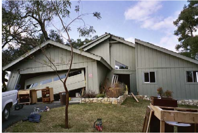
FIGURE 2-2 Atascadero, California, January 25, 2004. This home slid two feet off its foundation due to the 6.5 San Simeon earthquake. Photo by Dane Golden/FEMA News Photo.
