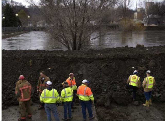
FIGURE 3-4 Valley City, North Dakota, April 13, 2009. Members of the U.S. Army Corps of Engineers inspect the site of a levee where severe seepage threatens the integrity of the levee in downtown Valley City, North Dakota. The Corps is working with city officials and the National Guard to ensure the safety of the levees in the town. Photo by Patsy Lynch/FEMA.
