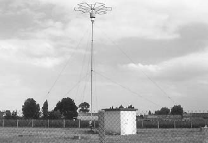
Figure 4-36. NDB nondirectional beacon. (Source: FAA)
