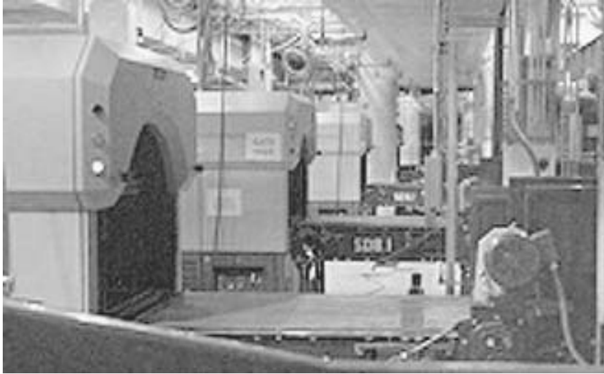
Figure 8-8. EDS machines located “in line” in baggage sorting areas. (Photo courtesy Boeing Corp.)
