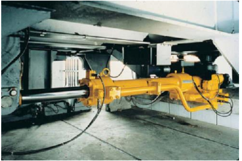
Plate 1 Active Control of Civil Structures. Actuator used in the Hybrid Mass Damper System in INTES.
