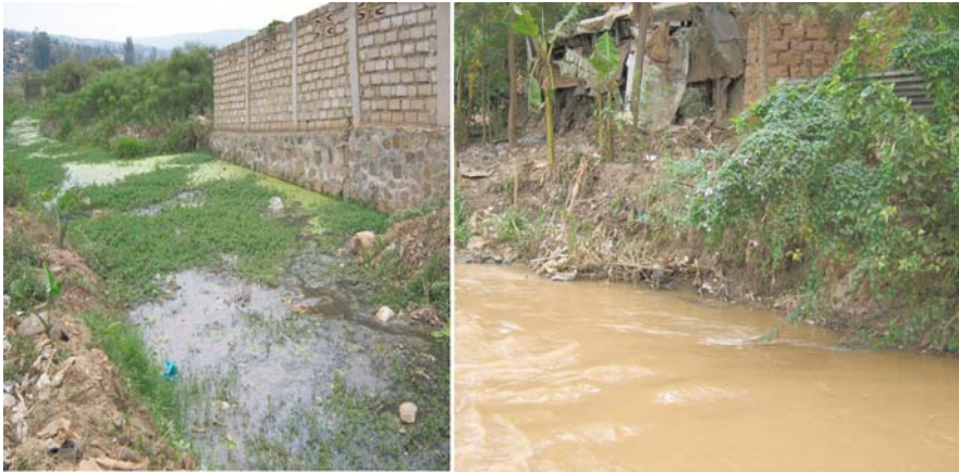
Fig. 6.15 Vulnerability of housing by location. Collapsed house in swampy area; A house near the river stream
