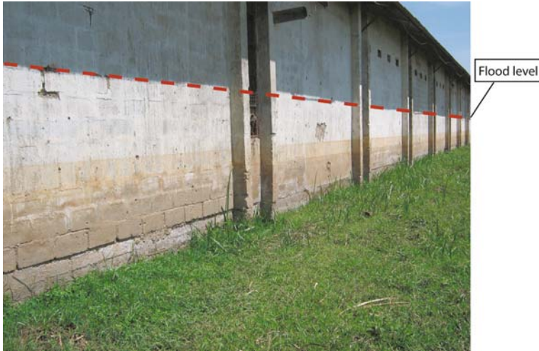
Fig. 6.5 Flood level observed in RWANTEXICO floods of April 2006 Source: Photo taken by Jean Pierre Bizimana, September 2006
