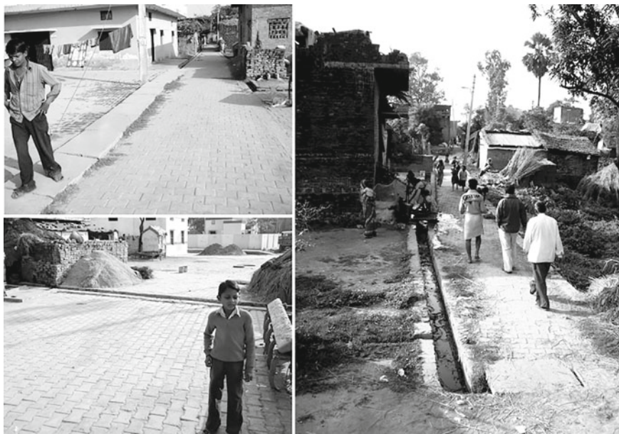
Fig. 4.13 Renovation of ward no. 5 in Siddarthnagar. Note Taken over by DUDA as part of the Kanshi Ram programme initiated by Mayawati, the predominantly SC ward no. 5 has been entirely renovated. It now has good quality road infrastructure, the roads and squares have been paved, nalas have been dug (some of which are covered) and new water pumps installed. Source Author
