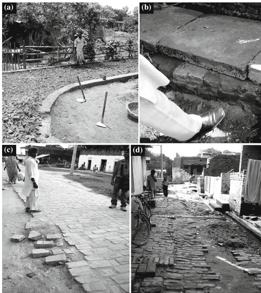
Fig. 4.12 The poor quality of the road infrastructure. Notes The misappropriation of funds on road and nalas construction projects undertaken by local building firms (a) reduces the quality of the infrastructure built. In (b), a disgruntled resident is kicking a nala recently constructed by the municipality in Siddarthnagar to demonstrate its fragility, which is due to the entrepreneur having scrimped on cement. The third photo (c), taken in Chandauli, shows a similar example: this is a newly paved street, but it is already beginning to break up. The last photo (d) shows one of many streets in Phulpur that is in an advanced stage of deterioration. Source Author
