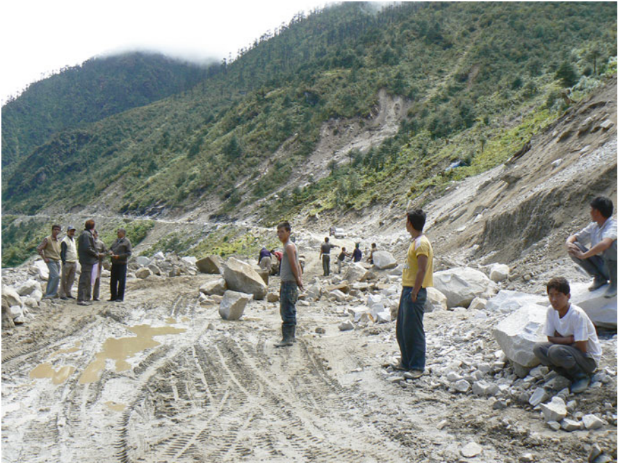
Fig. 1.4 Landslides occur at many locations on the road between the Arunachal highlands and Assam lowlands in the rainy season
