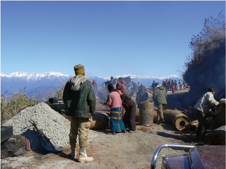
Fig. 1.2 Arunachal Himalaya, which divides the Dirang [rdi rang] area from the Tawang [rta wang/ dbang] area (background), and migrating workers from Nepal undertaking road construction
