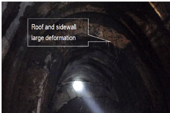
FIGURE 4.5 Roof and sidewall large deformation of the tunnel.
