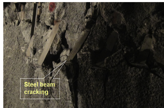
FIGURE 4.4 No. 20 I-beam steel distortion and cracking of the tunnel.
