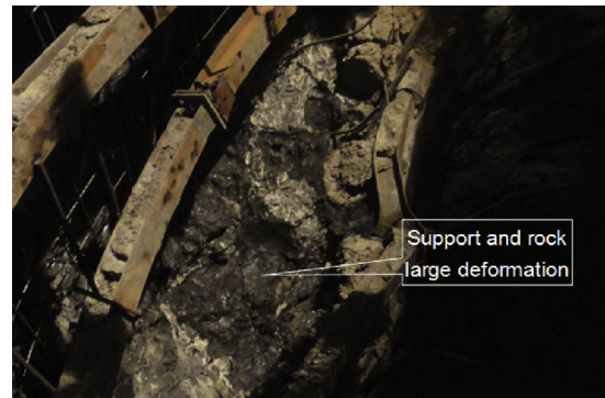
FIGURE 4.6 Large deformation of steel beam and the surrounding rock.
