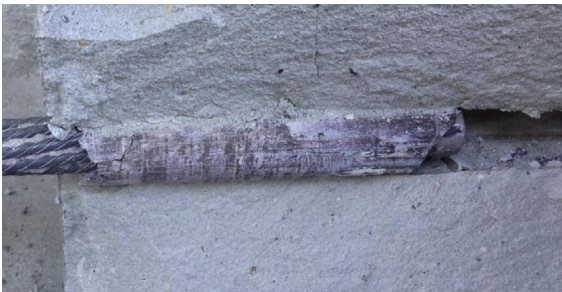
FIGURE 3.47 An example of failure of the cable at the grout/rock interface.
