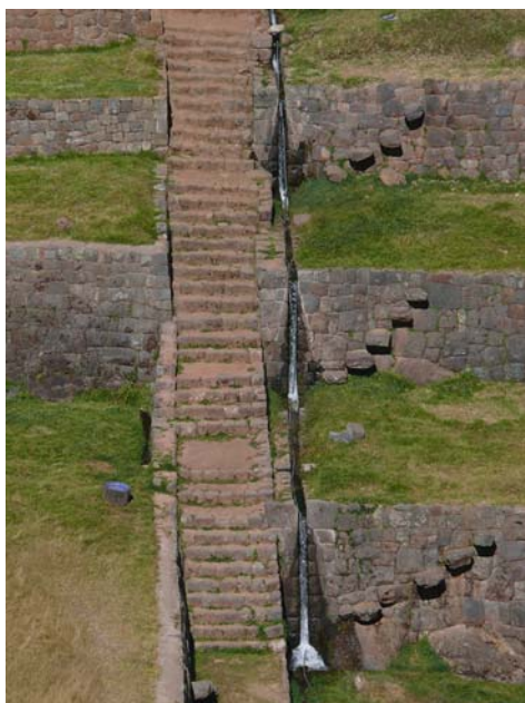
Fig. 9.22 Hydraulic drop structures near the middle of the central terraces in Tipon (photo copyright by Yuri Gorokhovich)
