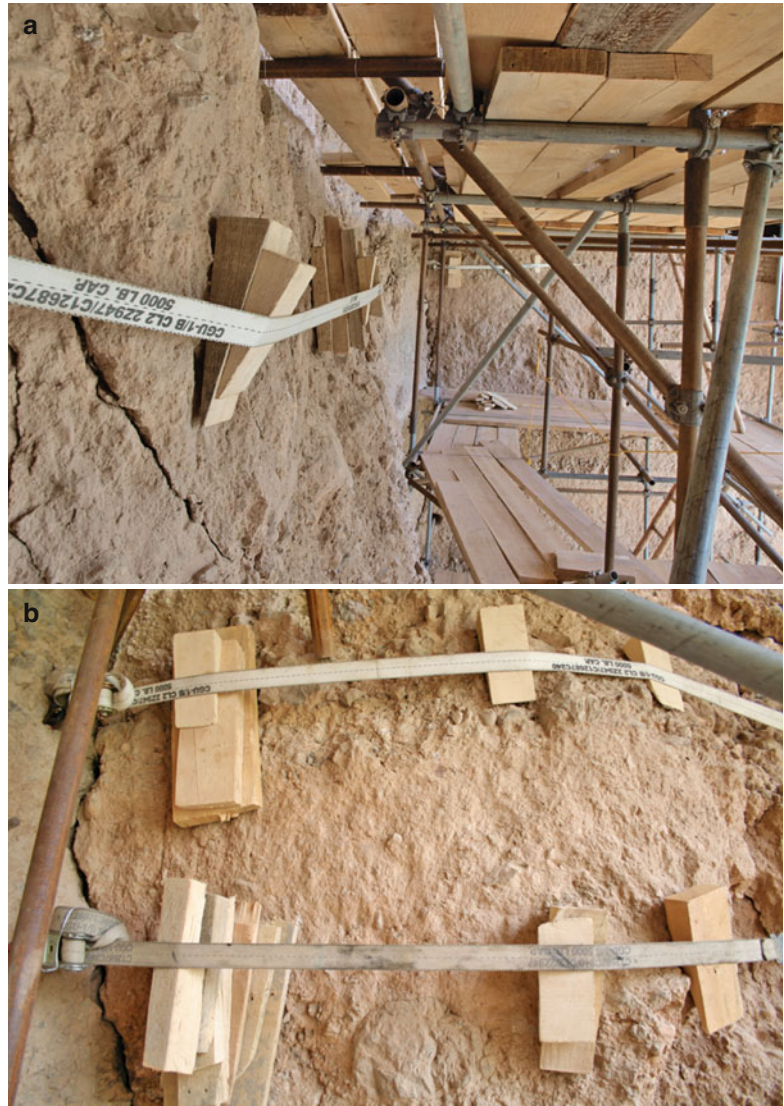
Fig. 13.12 (a–d) Temporary covering of the brittle parts at the Eastern Buddha by means of heavy duty tension belts as a first step of securing the back wall
