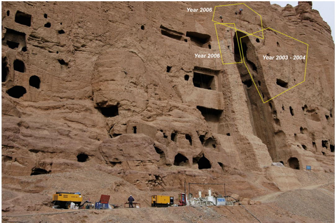
Fig. 11.4 Localization of the three areas of intervention in the Eastern Giant Buddha niche
