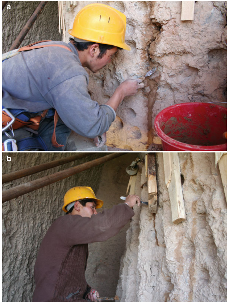
Fig. 13.13 (a, b) Sealing the cracks and backfilling step by step with mortar
