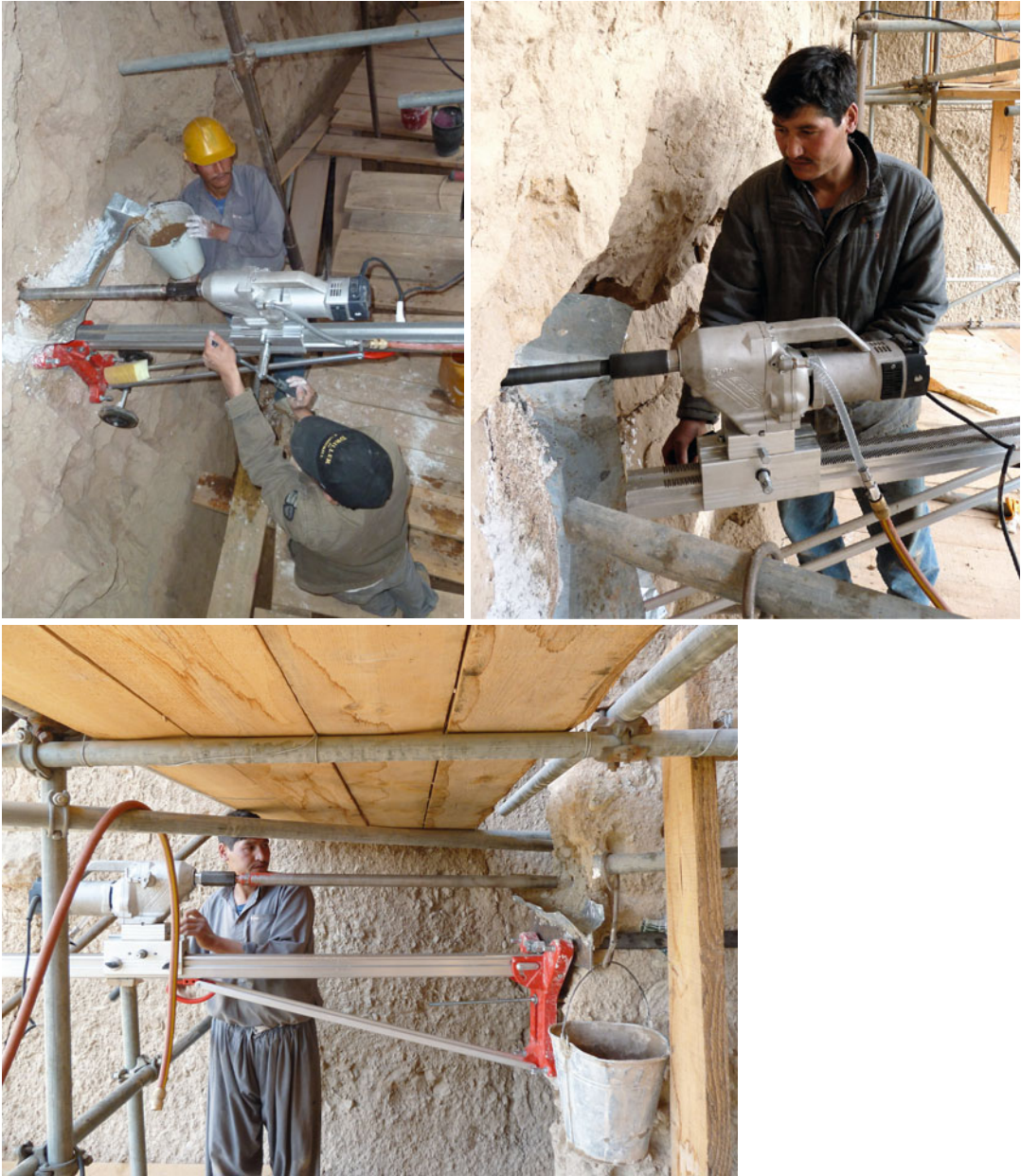
Figs. 13.16, 13.17, and 13.18 Diamond core head drilling in different situations. The water used for cooling is collected by a suitable folded panel in buckets, so the rock surface was protected of water
