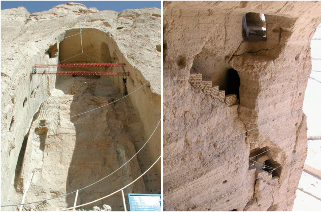
Fig. 11.6 The temporary beams ( left ) and steel cables ( right ) for the temporary support of upper eastern part of Eastern Giant Buddha niche
