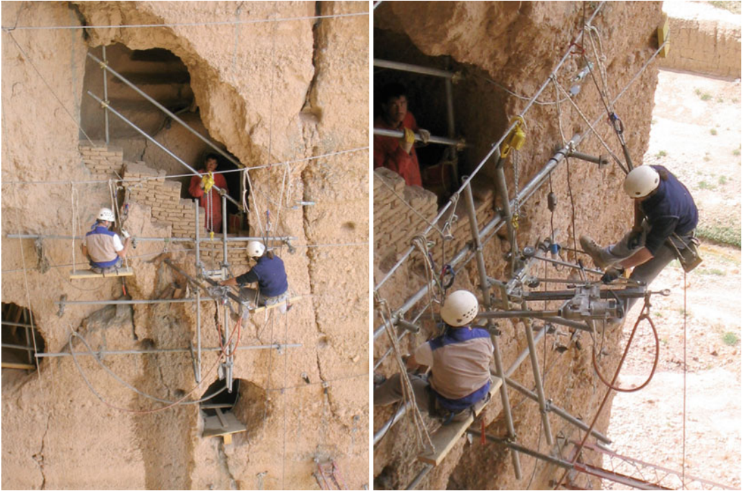
Fig. 11.15 Execution of nails with rotary machine and diamond head, at the inner side of the niche
