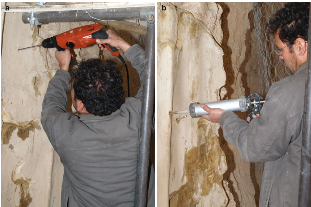
Fig. 13.7 (a, b) Original clay plaster fragments ( right side of the Eastern Buddha). Preparation for the setting of needles: Mirzai drilling a hole into an existing bullet hole
