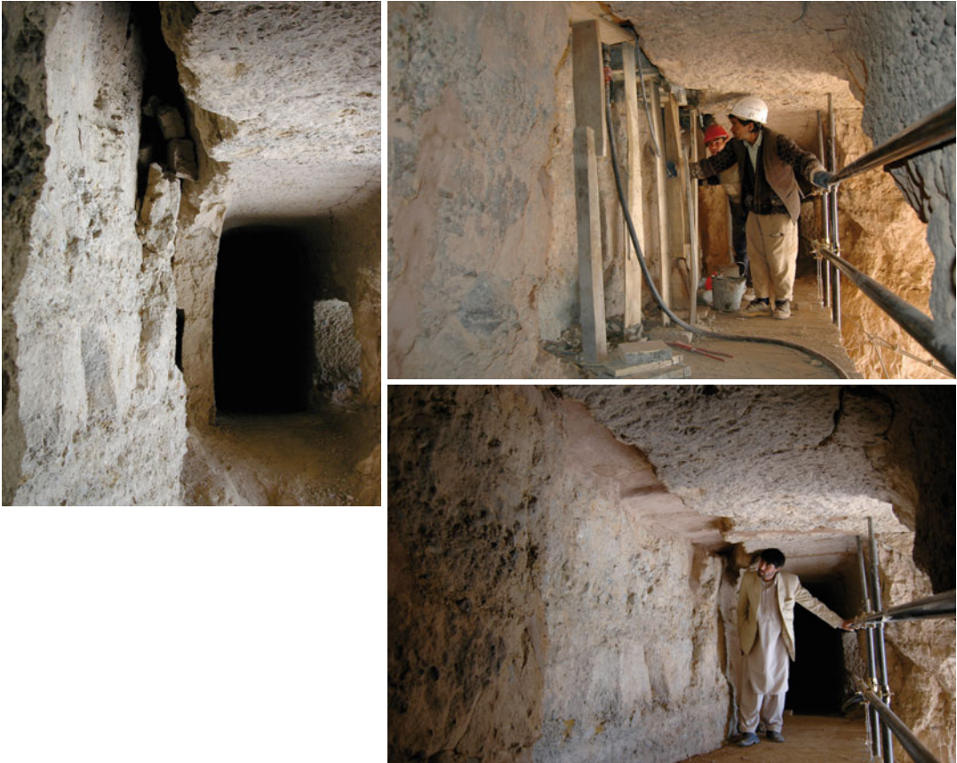
Fig. 11.39 ( The three figures ) The large crack in the corridor on the back side of the niche before, during, and after the grouting
