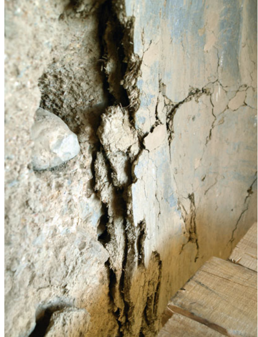
Fig. 13.6 Three layers of clay plaster, partly detached from one another
