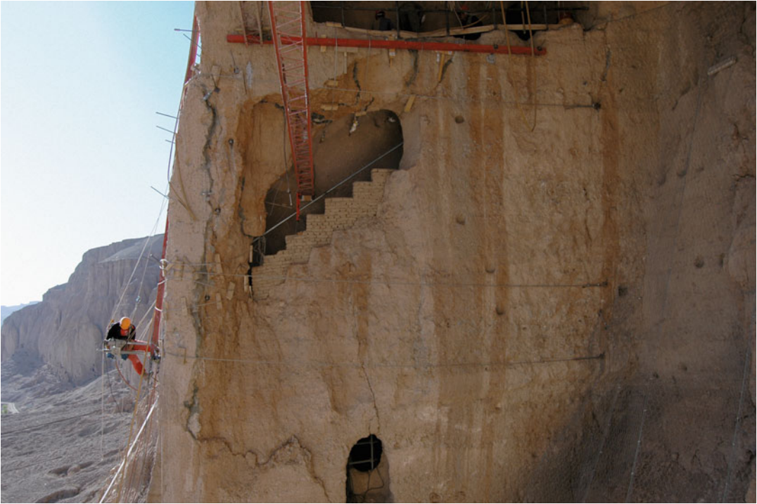
Fig. 11.27 Drilling for nails on the west side, with intermediate power machine and diamond head
