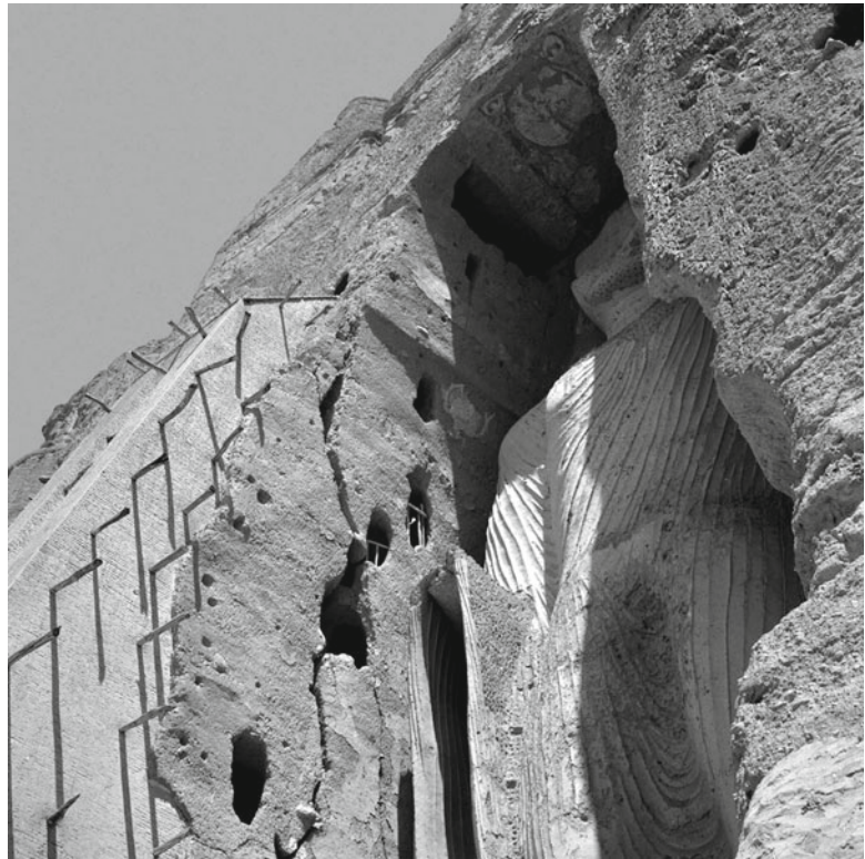
Fig. 9.2 The buttress and the most external part of the cliff showing the large crack and the detached block, which needs support. It is not clear whether the crack was moving at the time of the picture or not. Nevertheless, the crack was detected as slightly open in the 2002 survey by the authors (Photo A. Bruno, Sept. 1960)
