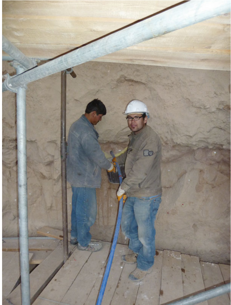
Fig. 13.19 Filling in the mortar in the bore holes. After filling up the fissures with mortar, a second drilling had to be done to position the anchors
