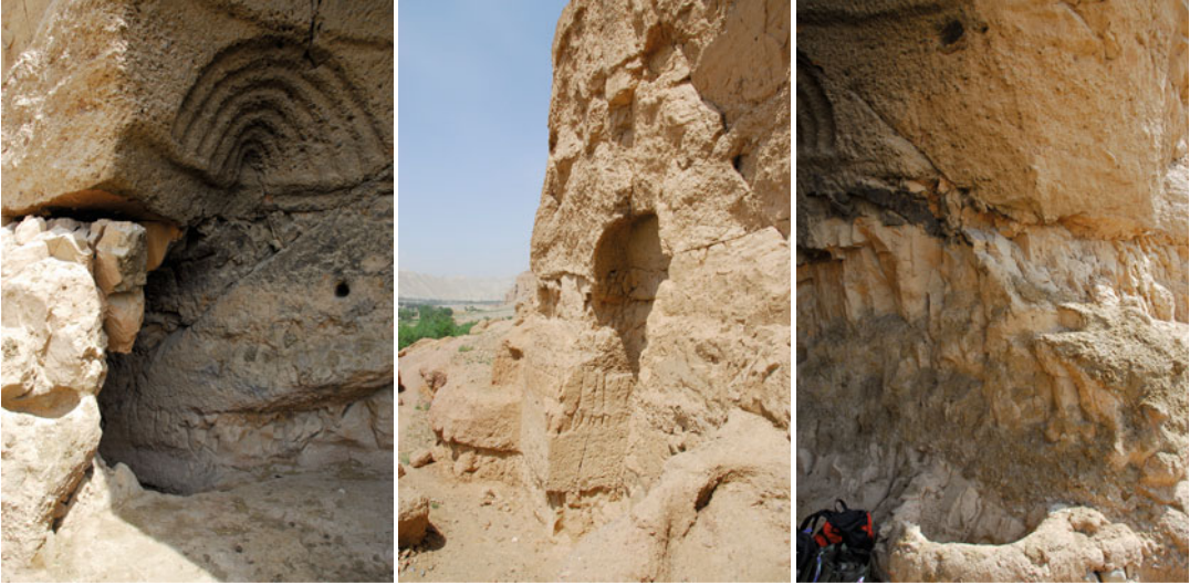
Fig. 5.34 Example of wedge failure potential area in the east side of the cliff
