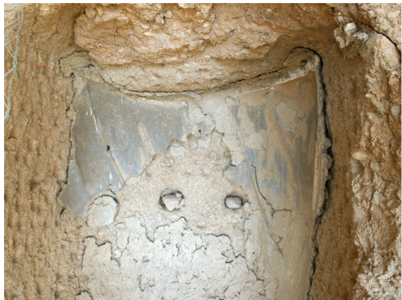
Figs. 13.2 and 13.3 Eastern Buddha: remains of clay plaster on the left, with lapis lazuli. Photo shows condition before treatment. All fragments are slightly detached from the rock face and are only kept together by being wedged on the left and right with the “clay-stone burling”
