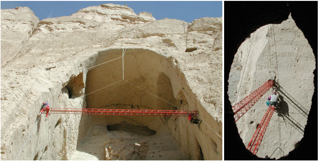
Fig. 11.10 Installation of temporary struts. Note that during the installation, the strut is fixed on top of the cliff in the safe zone
