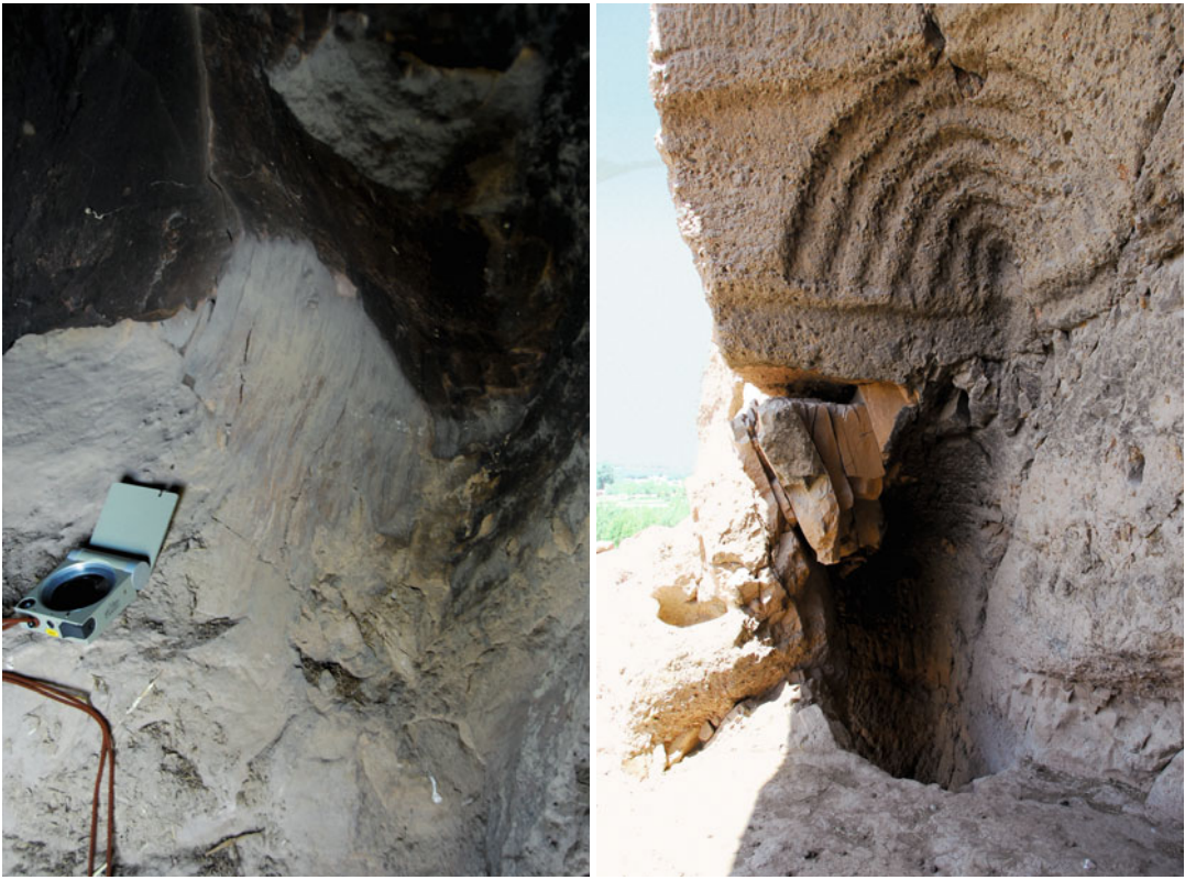
Fig. 5.32 Fault surface with evidence of stress ( left ) and persistent discontinuity where potential planar sliding can develop ( right )
