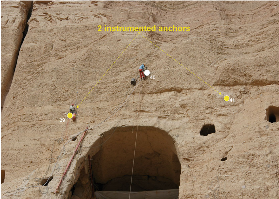
Fig. 11.29 Position of anchors on the top of niche. The yellow ones are monitored with 10 strain gauges
