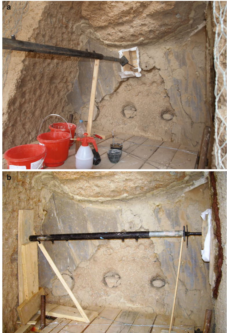
Fig. 13.8 (a–c) Bonding of the clay plaster fragments. By means of a splaying apparatus, pressure is carefully put on the clay plaster fragments. In most cases this apparatus was hinged to the scaffold. The surface of this apparatus was adapted to the texture of the clay plaster and was made of small wooden boards. On the left underneath the arm hole
