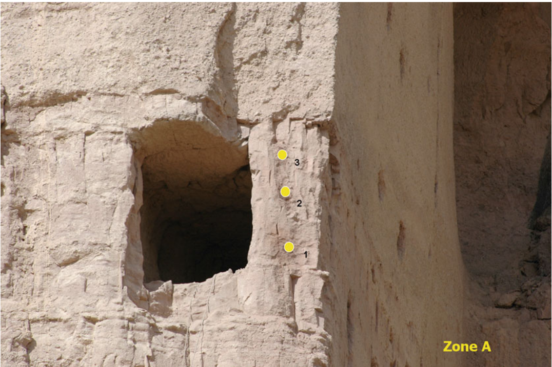
Fig. 11.43 Position of nails in the unstable small rock masses at middle level of the niche
