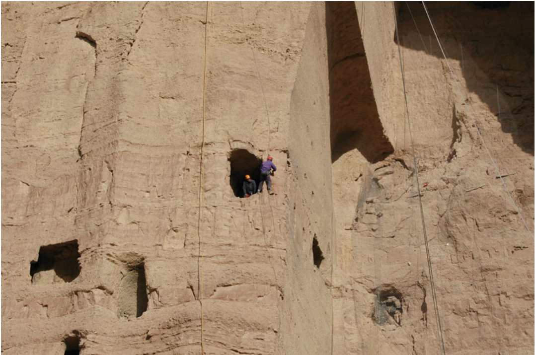
Fig. 11.41 Preparation for consolidating the potential small rock fall at middle level of the niche
