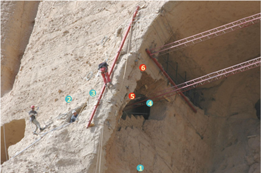
Fig. 11.21 The location of potentiometric crack gauges for discontinuity monitoring and alarm; external sensors are in green and red are internal to the cave
