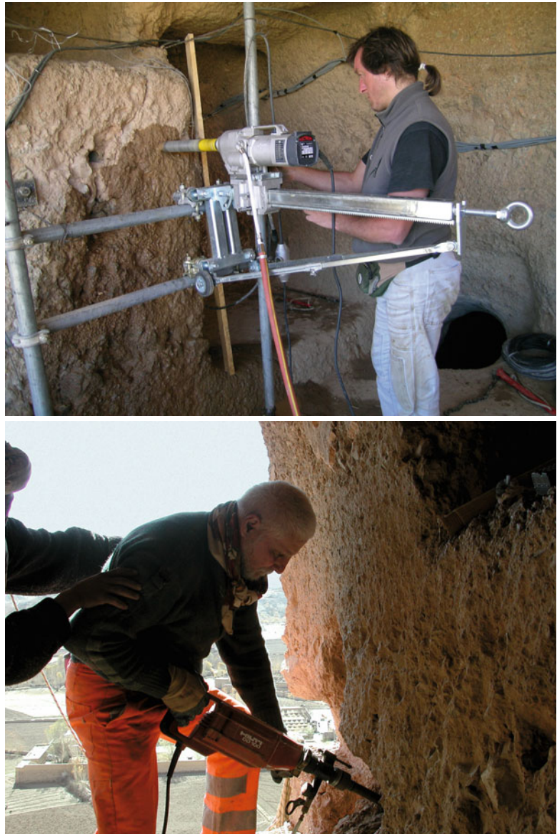
Fig. 11.16 Detail of execution of nails from inside the caves by means of small and very small rotary machines and diamond heads
