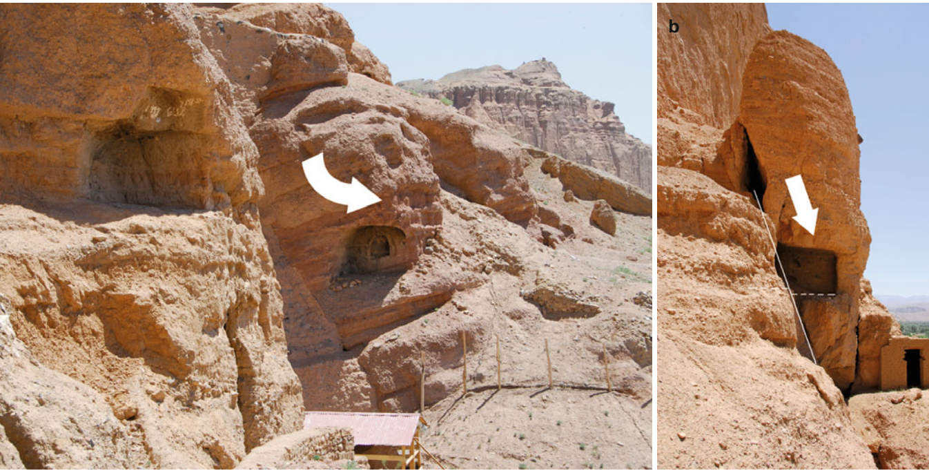
Fig. 5.18 Cave's ground floor tilted after a rock slide east of Western Giant Buddha ( left ) and a cave displaced by a rock slide's plane west of Eastern Giant Buddha ( right )
