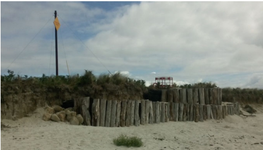
Fig. 5.47 Reinforced telephone cable junction on Tresco, February 2014
