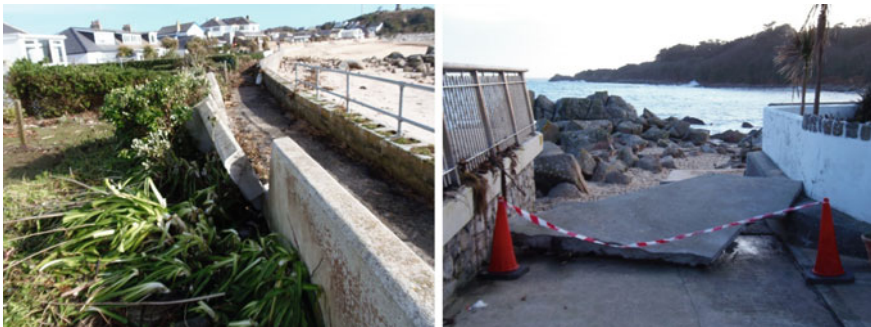
Fig. 5.7 Damaged sea wall and slipway at Porthcressa, February 15, 2014 ( Source both, A. Martin, private photograph, 15/02/2014 )
