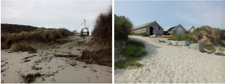
Fig. 5.48 Damaged slipway after storms ( left ), March 2014; the same slipway repaired in July 2014 ( right )
