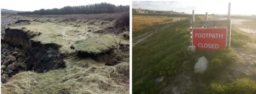
Fig. 5.14 Erosion on St Agnes ( left ; February 2014); closed footpath due to erosion ( right ; September 2015)
