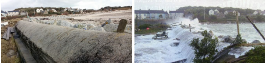
Fig. 5.13 Seawall on Bryher built in the 1960s ( left , February 2014), overtopped by a surge in 2014 ( right , source R. Pearce, private photograph, February 2014)
