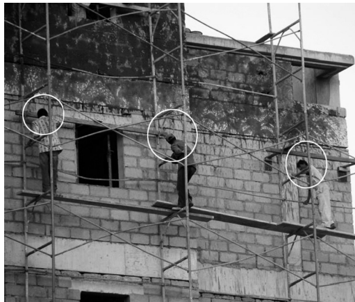
Figure 8.3 Unsafe construction site, in addition to non-safety precautions by construction workers.
