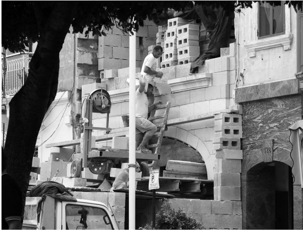
Figure 8.4 Unsafe manoeuvres and non-safety precautions by construction workers on a ladder.
