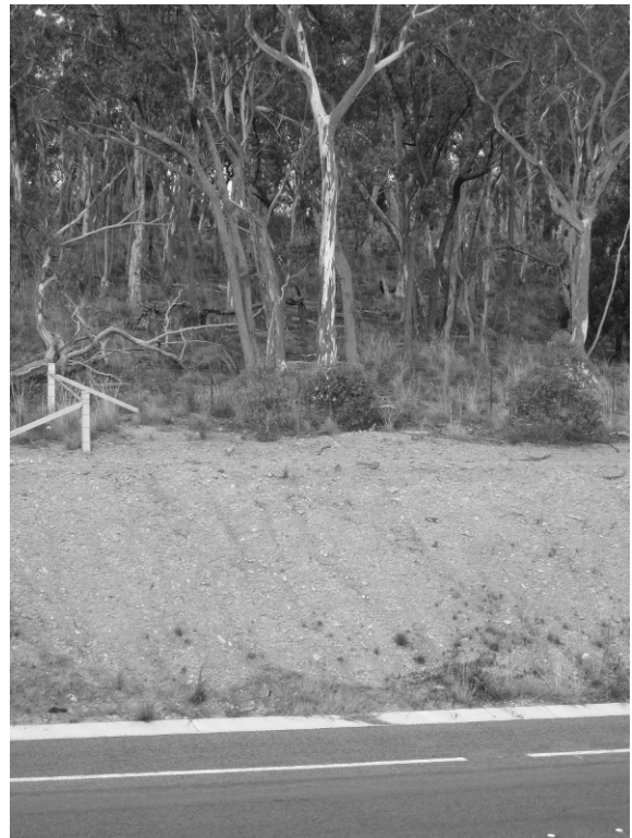
FIGURE 12.2. A road verge slope showing signs of sheet and rill erosion caused by excessive overland flows from above the roadway. Flows have also washed away the mulch that was originally applied to this slope.
