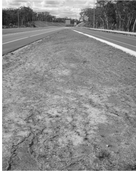
FIGURE 12.6. An “island” road verge where a surface mulch of fine stones has failed to resist erosion by overland flows. Note the wash of surface litter and sediments.
