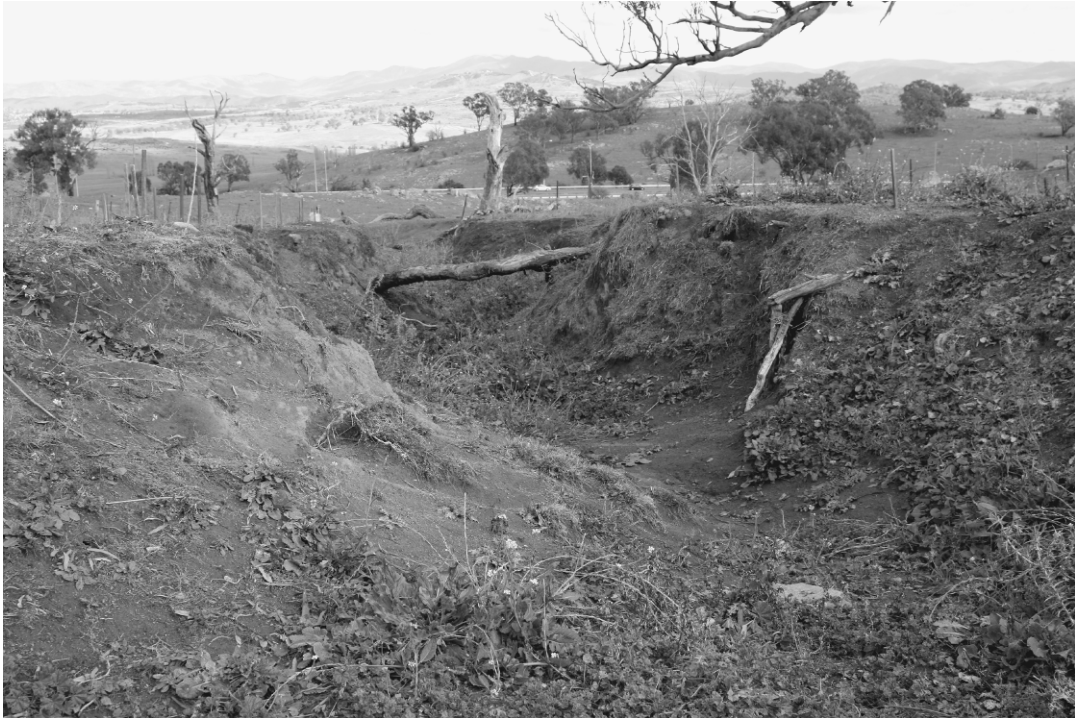
FIGURE 11.6. An example of an eroding and weedy drainage line on a hillslope pasture in former ACT farmland.
