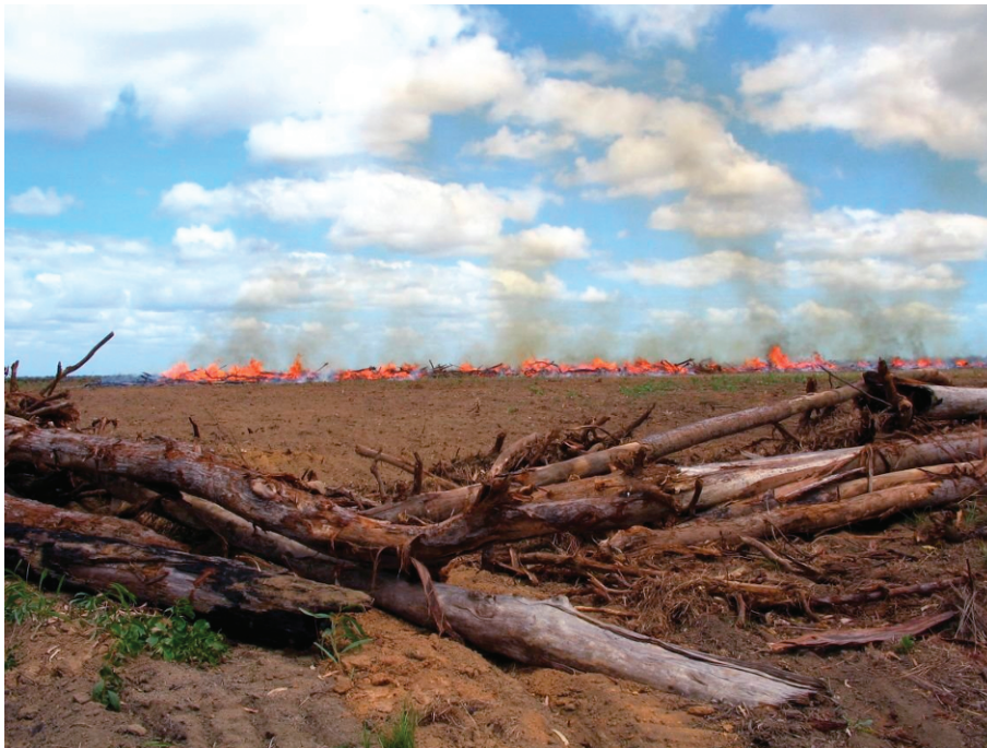
PLATE 4.2. Landscape being prepared for mining bauxite by pushing open forest vegetation into windrows that are burnt when dry. Photograph courtesy of Sue Gould.
