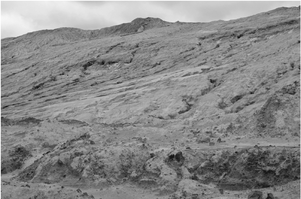
FIGURE 7.6. Overflow from the top of a TSF (at top right) has eroded the wall, carrying tailings off the site.
