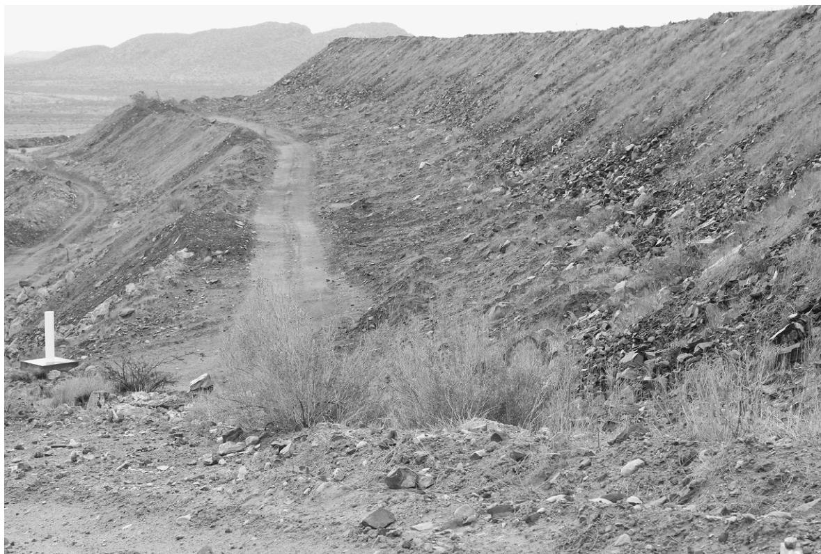
FIGURE 7.2. Stepped walls of a tailings storage facility built from dry tailings and covered with nonreactive waste rock.
