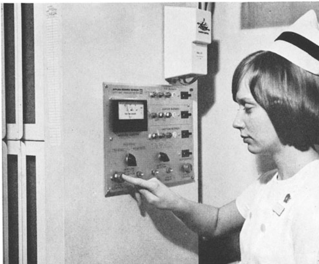
Fig. 6. Controls for lighting and air flow
