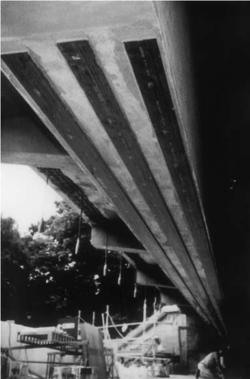
FIGURE 39.4 Plate bonding on the soffit of a bridge (photograph by kind permission of Sika Ltd, Welwyn Garden City, Herts, UK).
