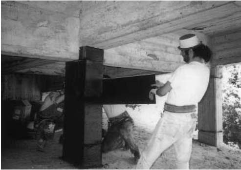
FIGURE 39.5 The use of REPLARK to wrap a column with carbon fibre polymer composite (photograph by kind permission of Sumitomo Corporation (UK) London).
