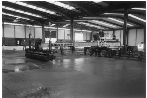
FIGURE 43.4 Laser-screed machine placing a steel fibre-reinforced concrete floor (by permission of Bekaert Building Products).
