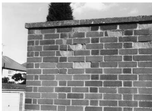
FIGURE 33.3 Erosion due to frost attack.
