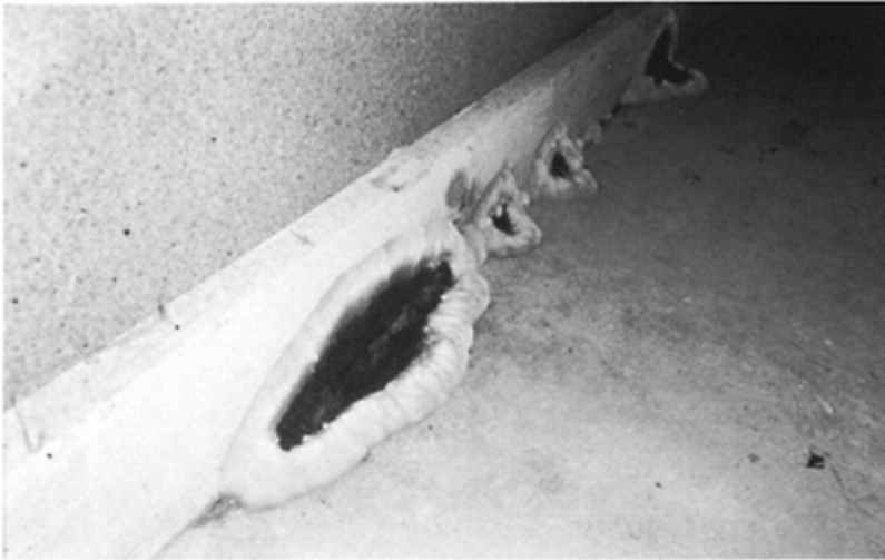
Figure 12.3 Fruit bodies of the dry rot fungus in a floor construction.
