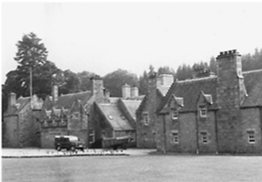
Crow steps leading to water penetration as a result of poor flashing.
