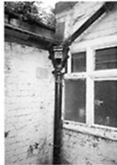
Over-discharge and blocked drainage leading to vegetative growth.
