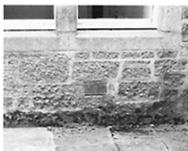
Ventilation of the floor void (floor ventilators).
