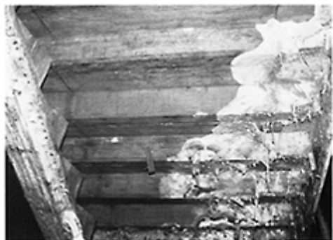
S. lacrymans (dry rot) mycelium and strands under stairs.
