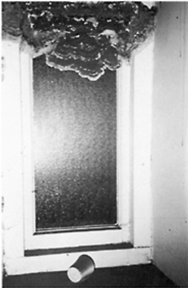
S. lacrymans (dry rot) fruiting body at the top of the window-frame with dry rot spores on the lower window-sill.
