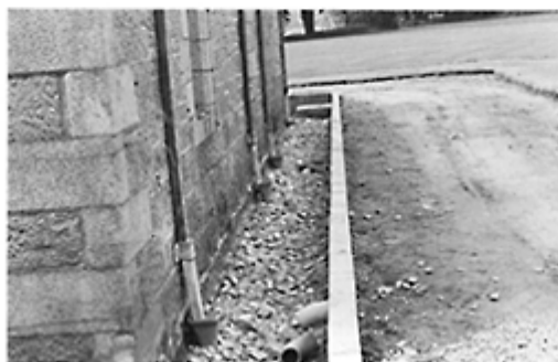
Dry line area (French drain) to lower ground level against external wall.
