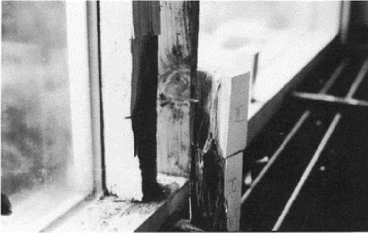
Figure 12.2 Modern window construction showing decay.
