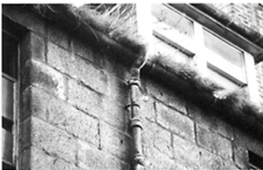
Extensive growth of vegetation due to blocked guttering and downpipe.
