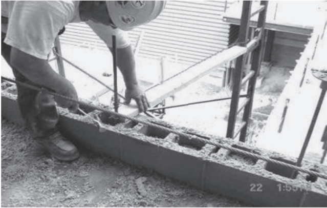
Protection often removed to work
