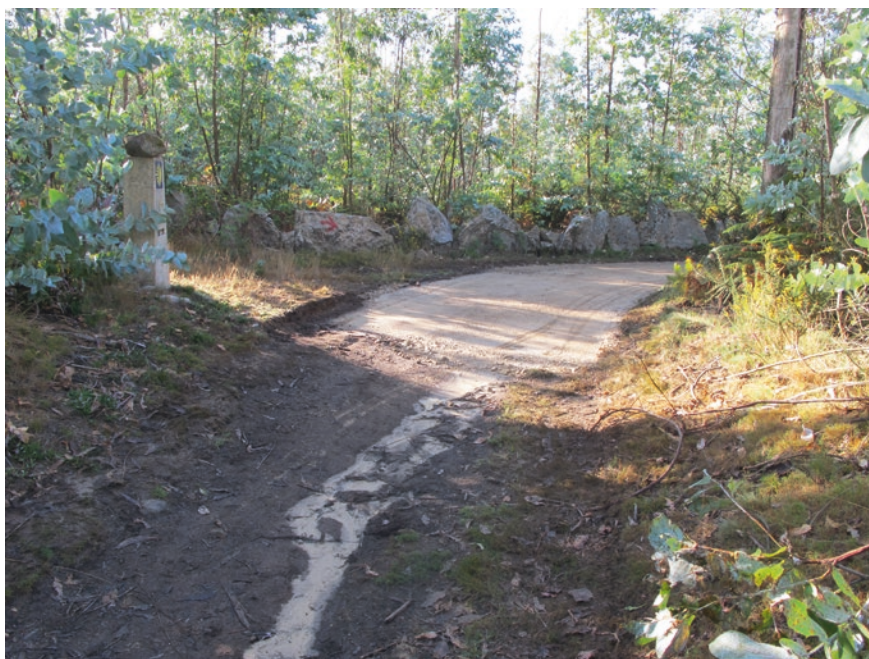
Fig. 4.7 Work being done by the state-owned company Tragsa in 2010 on the section of the Camino to Finisterre that passes through Dumbría. Source Cristina Sánchez-Carretero
