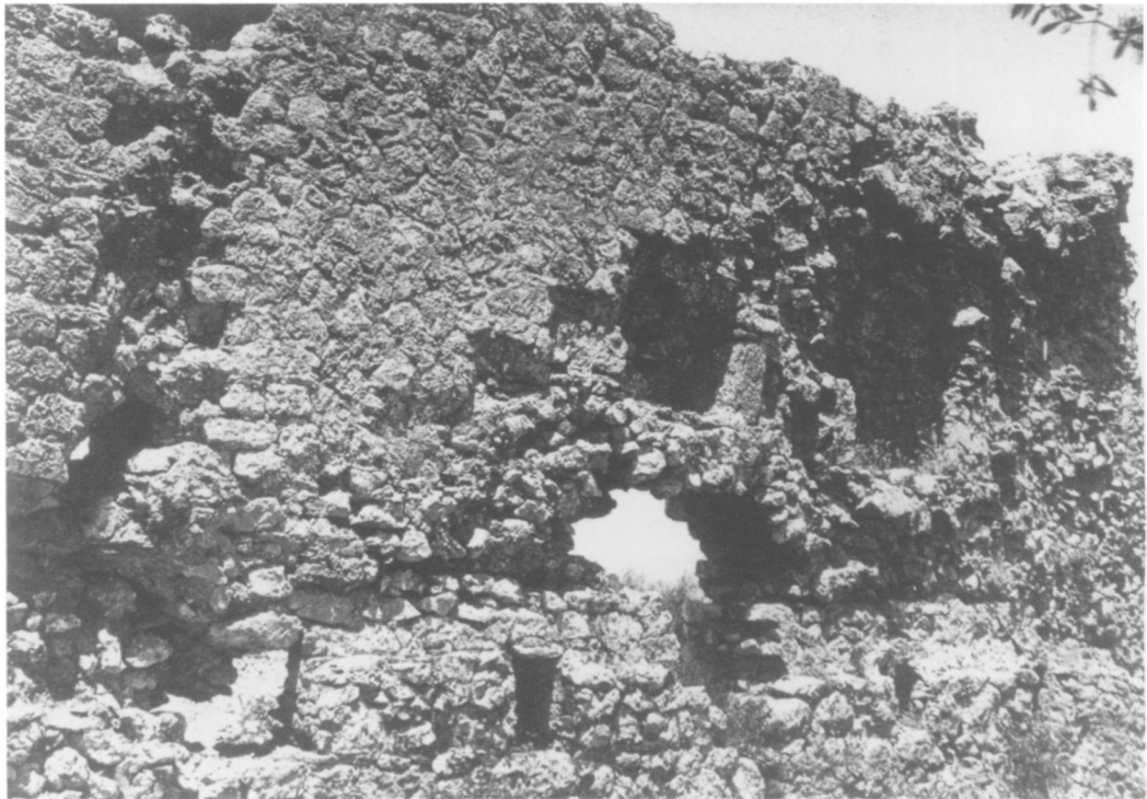
PLATE 240. Basilica, stair to the platform above the ambulatory, print on the NW wall of Curia III
