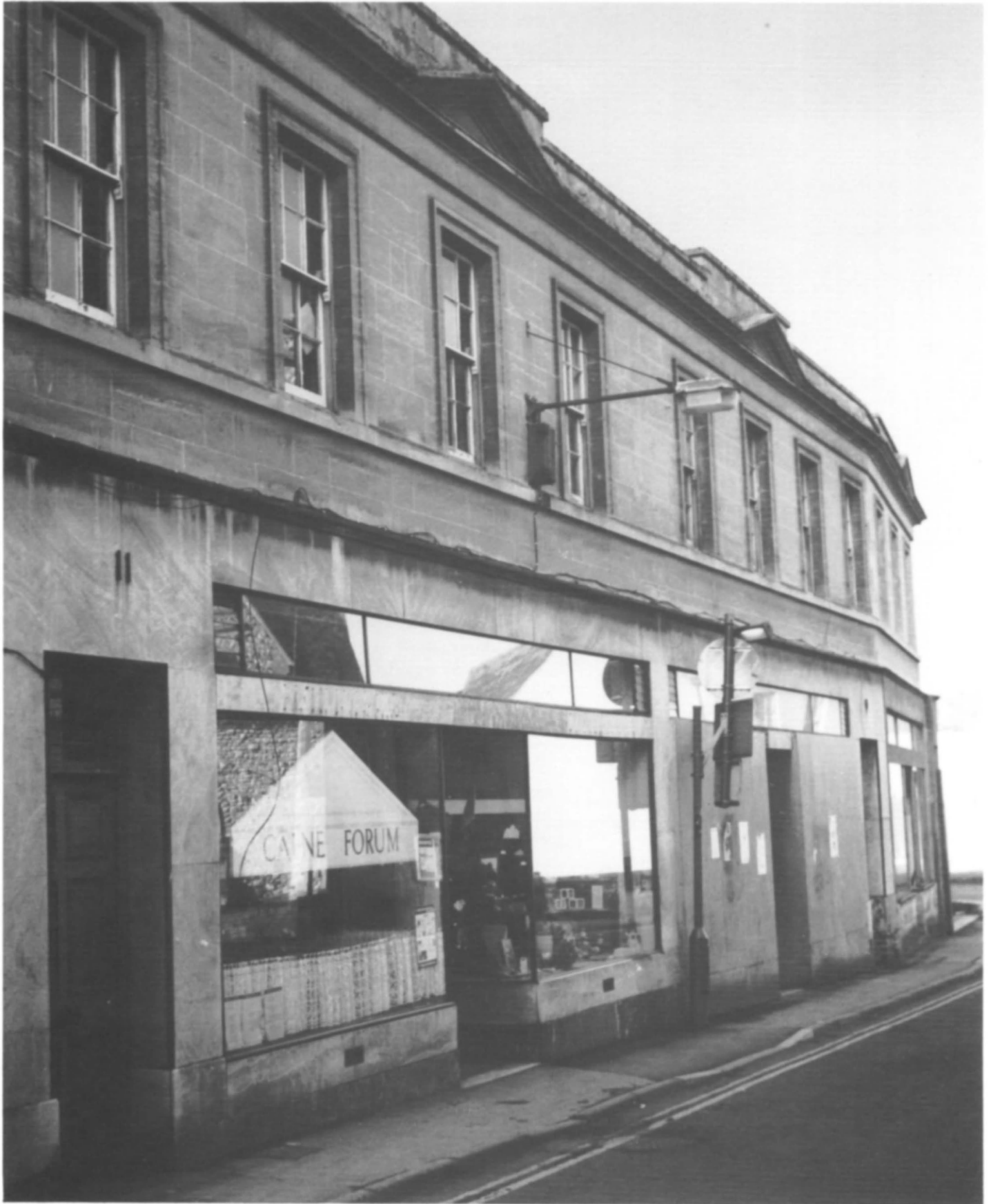
Fig 37 Whilst this terrace in Calne waited for rehabilitation in 1987, the temporary use of one unit by a charity shop was of benefit to the building and the surroundings, in contrast to the boarded up unit next to it
