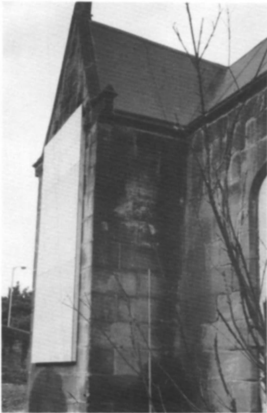
Fig 101 Brandling Station, Felling: temporary roofing and boarding up in 1975 (photo: Tyne & Wear County Council)
