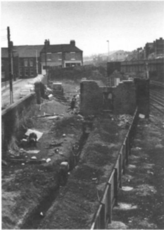
Fig 103 Brandling Station, Felling: in spite of temporary repairs, the full rehabilitation in 1978 involved demolition of the roof and west gables (photo: Tyne & Wear County Council)
