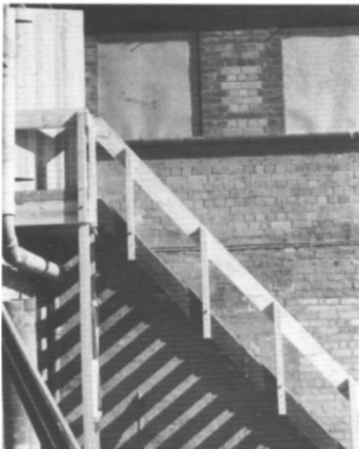
Fig 10 A temporary stairway leading to otherwise inaccessible parts of Maw's Tileworks, Ironbridge (photo: A T Herbert)
