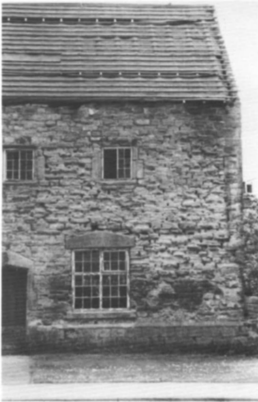
Fig 25 Complete lack of protection at eaves level in 1981 resulted in disastrous erosion of the stonework at Barlborough Old Hall (photo: Bob Hawkins)
