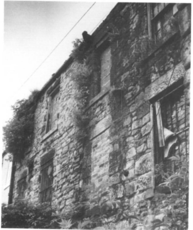
Fig 28 Plants flourishing in weak mortar joints with an ample water supply from broken gutters
