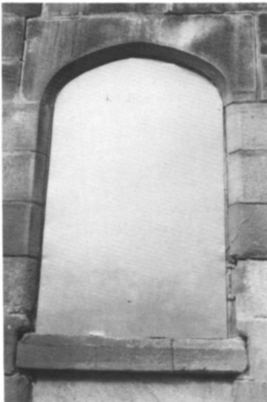
Fig 102 Brandling Station, Felling: a neatly sealed window (photo: Tyne & Wear County Council)
