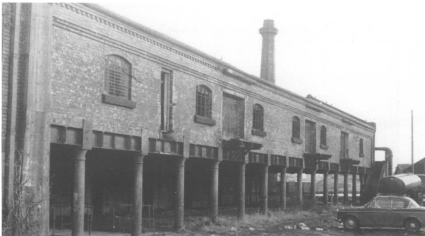
Fig 120 Island Warehouse, Ellesmere Port: in 1974 the building was open to vandals and the canal arm filled with debris (photo: The Boat Museum Trust)
