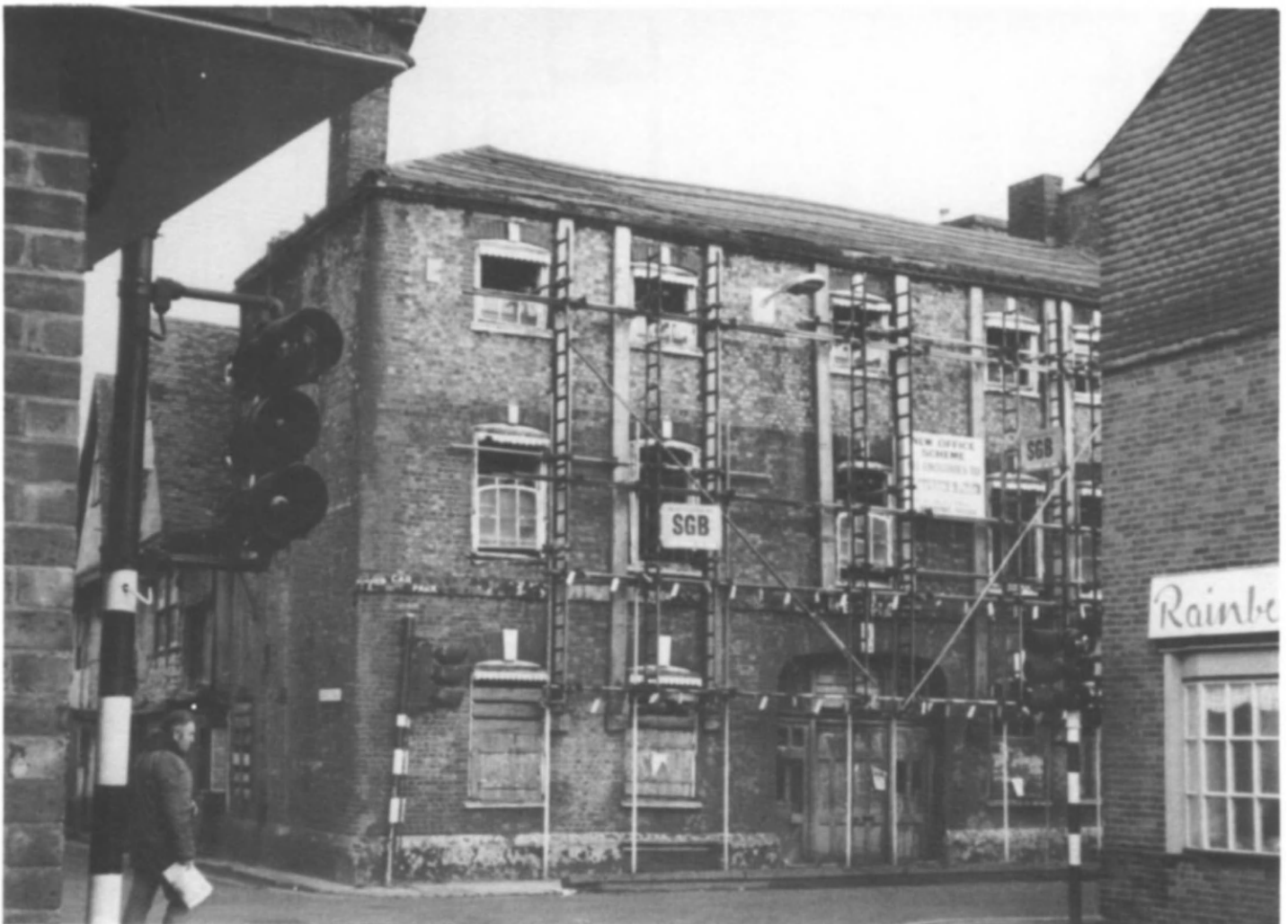
Fig 41 The Lamb Inn before repair in 1978, with support scaffold in position (photo: Colin Bridger)
