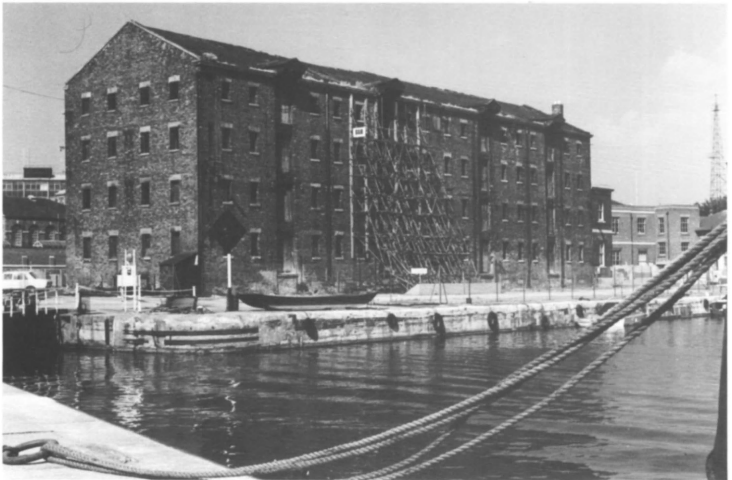
Fig 8 Support for brickwork which was pushed out by a fallen truss in the North Warehouse, Gloucester Docks; this scaffolding was hired initially for three years but remained in place from 1975 to 1985 (photo: Richard Parsons)
