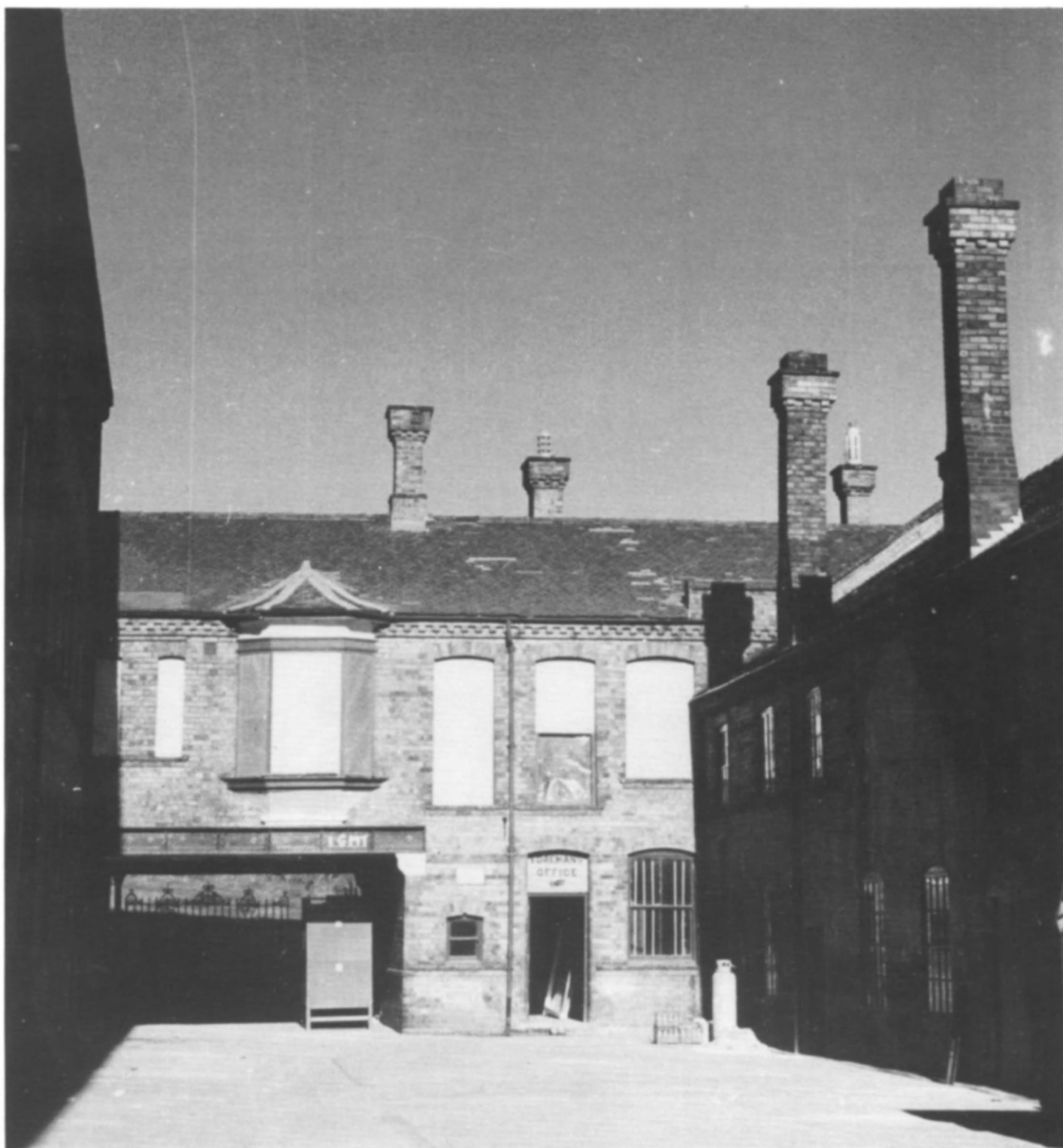
Fig 133 Maw's Tileworks, Ironbridge: the office building under emergency repair (photo: A T Herbert)
