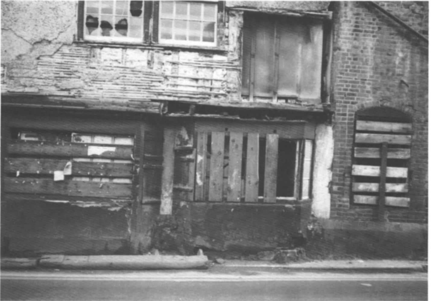
Fig 18 Boarding which can be levered off is ineffective; inadequate traffic protection has resulted in damage from high-sided vehicles (photo: Ann Bridger)
