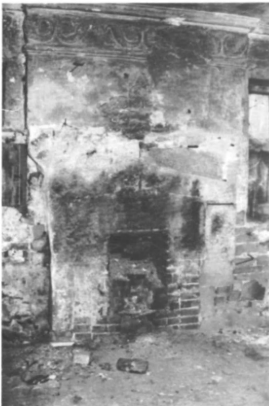
Fig 31 Seventeenth-century plasterwork at Barlborough Old Hall threatened by damp penetration from rubbish blocking the flue behind it (photo: Bob Hawkins)
