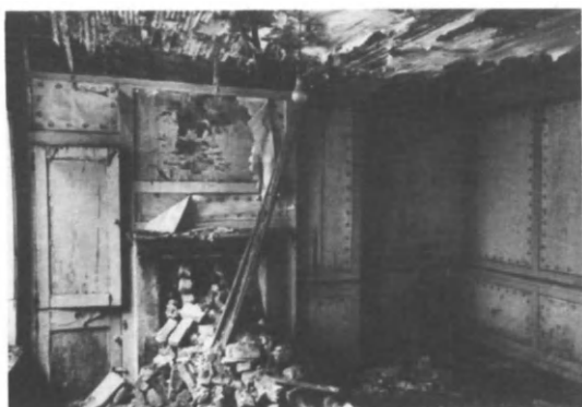
Fig 49 5-7 Elder Street, Spitalfields: an example of the condition of the original panelling which was saved as part of the emergency repairs (photo: Julian Harrap Architects)
