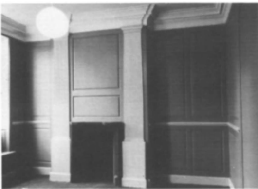
Fig 58 Arkwright House, Preston: meticulously repaired panelling and a newly designed fire surround (photo: Architectural Heritage Fund)
