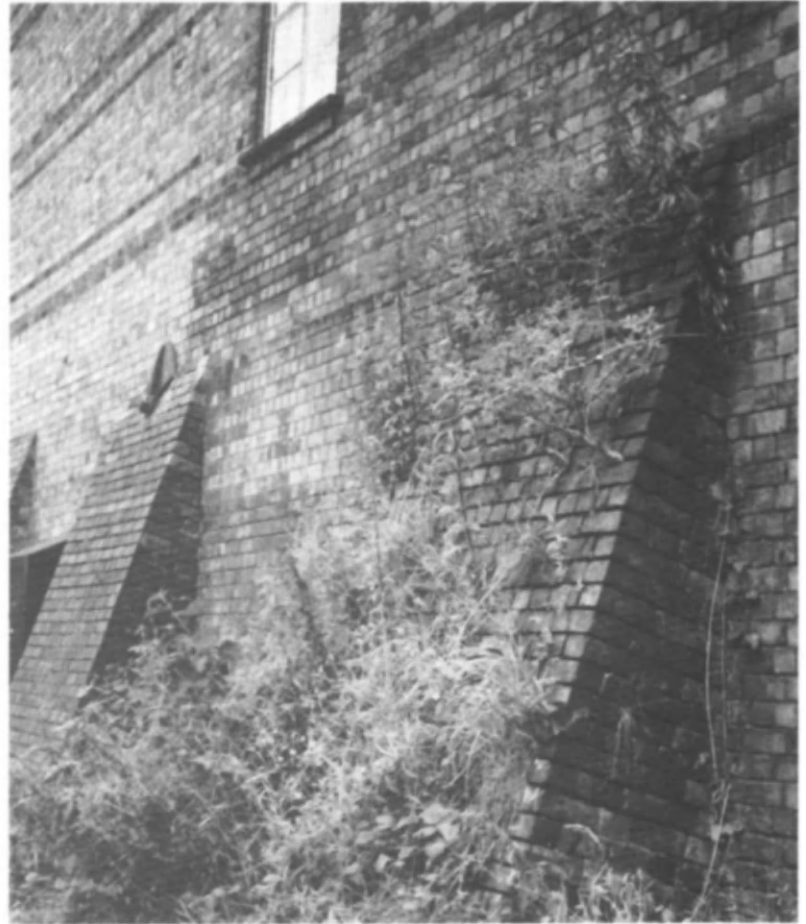
Fig 29 Sloping surfaces harbour seeds in brick joints leading to a risk of disintegration from strongly growing plant roots
