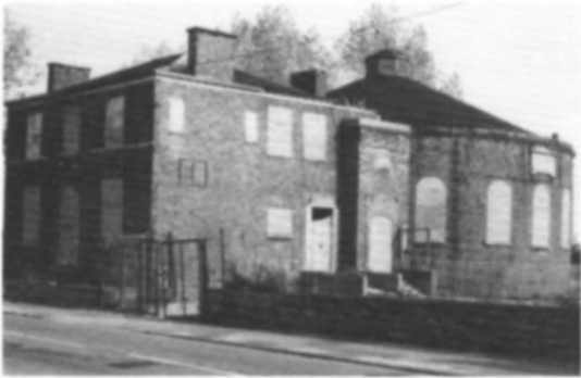
Fig 15 The Roundhouse Chapel, Manchester, was very strongly protected in 1978 while waiting for a new use, but vandals penetrated the structure itself, finding the old masonry weaker than the new (photo: The North West Civic Trust)
