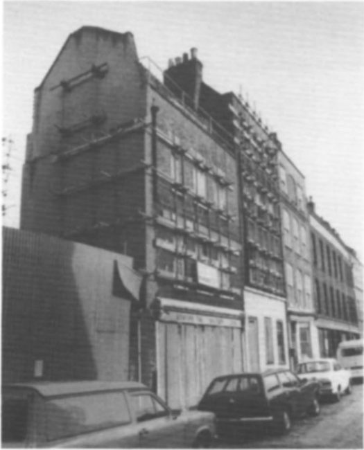
Fig 7 Gable and front elevation of 17 Folegate Street, Spitalfields, tied to an internal scaffold structure (photo: Anthony Richardson)
