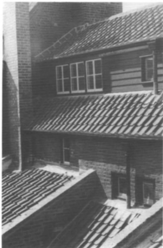
Fig 51 5-7 Elder Street, Spitalfields: the unusual roof formation giving rear light to the weaver's loft, rebuilt with original pantiles (photo: Julian Harrap Architects)
