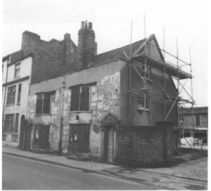
Fig 65 Gillygate, York: numbers 23 and 25; work beginning in 1982 after six years of temporary repair (photo: York City Council)
