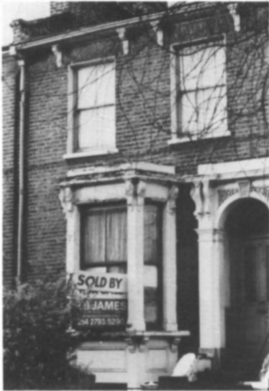
Fig 6 These garlanded corbels broke into pieces when the rotted bay was taken down for rebuilding; enough pieces were saved and reassembled to make a mould for replacements
