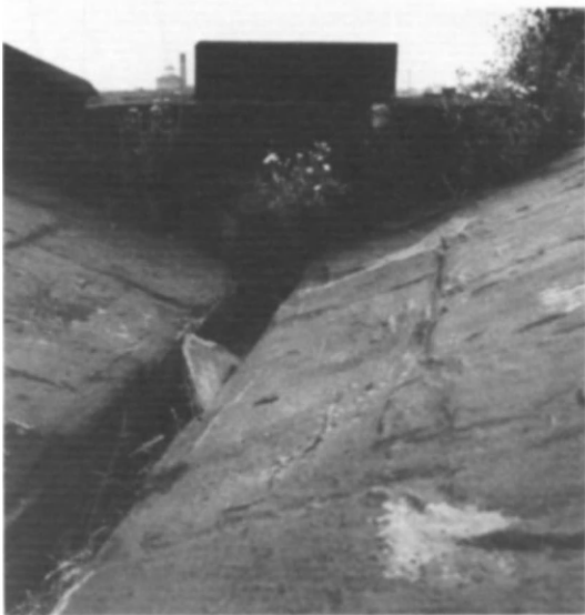
Fig 97 Warehouse, Liverpool Road Station, Manchester: the temporary roofing was intended to last five years, but after seven years it was failing
