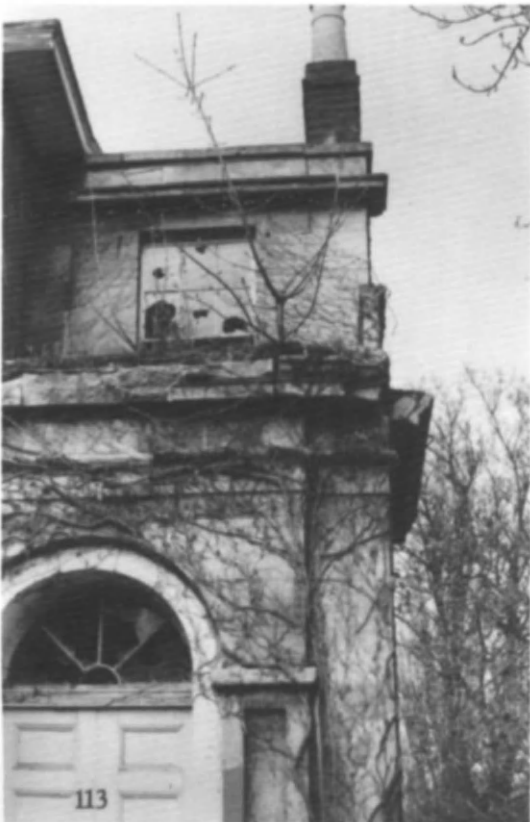
Fig 86 Bath Road, Cheltenham: number 113, overwhelmed with vegetation, and progressively losing the finely detailed stonework (photo: Cheltenham Borough Council)
