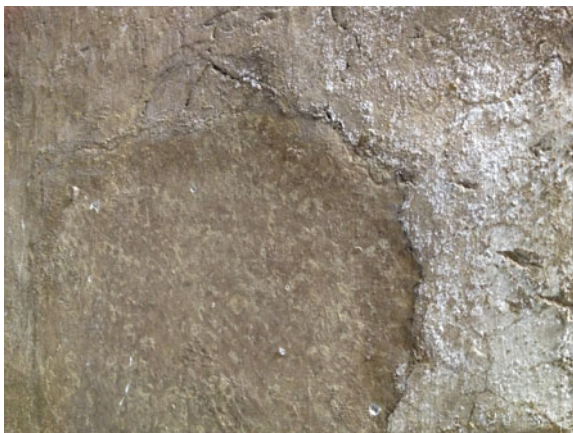
Fig. 9 White efflorescences are concentrated alongside the border of a patch which is composed by a different cement mix respect to the surrounding matrix
