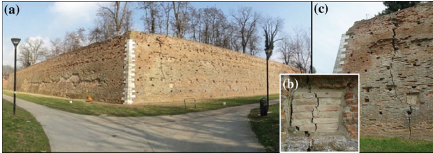
Fig. 2 a The tip of the bastion of Sant'Antonio and b, c detail of one of the major cracks
