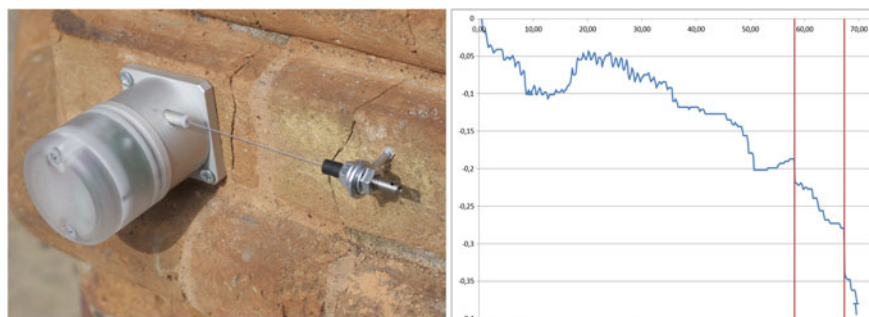
Fig. 3 When the damage mechanism is well understood, even very small, single point instruments (in the picture, one by Fiama srl, Parma) can allow to precisely control the evolution of cracks and to check the reaction of the building in case of singular events (in this case: earthquakes)
