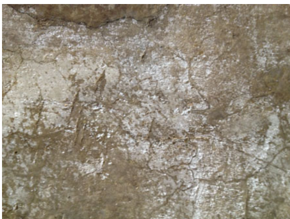
Fig. 10 White efflorescences are spread all over the surface but the patches
