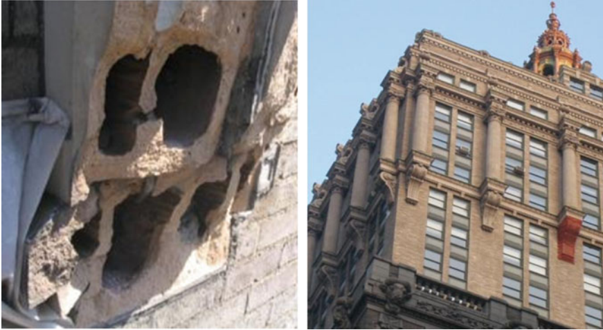
Fig. 3 Fractured terra-cotta bracket ( left ); brackets are located below the three-storey tall columns at the 28th floor of 230 park avenue, New York City ( right )
