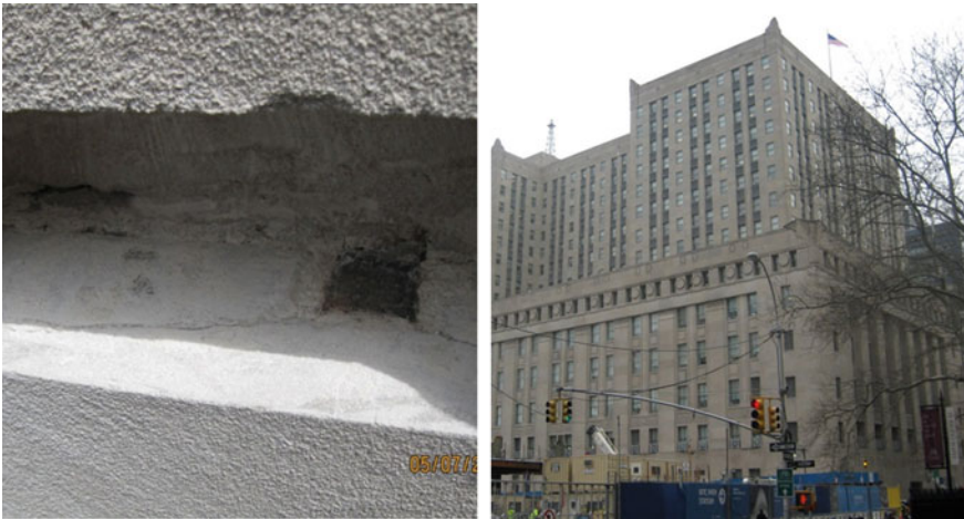
Fig. 4 A crack, originated by the corroded steel cramp and exposed by the removal of the adjacent stone unit, is visible at the cut line of the probe but not yet visible on face of the stone ( left ). Limestone façades of the office building ( right )
