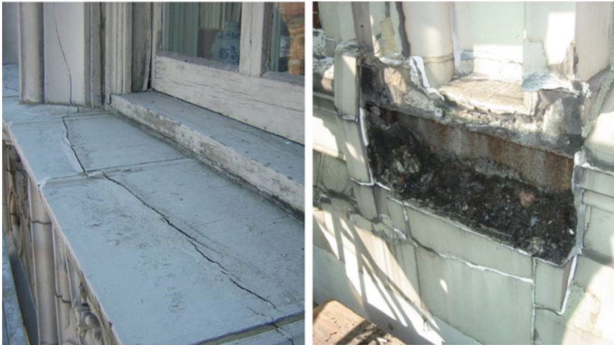
Fig. 2 Upper west side building. Fractured terra-cotta sill: cracking propagates along the entire length of the sill and up into the vertical pier ( left ). Extreme deterioration of terra-cotta ashlars due to the corrosion of the steel beam behind them ( right )
