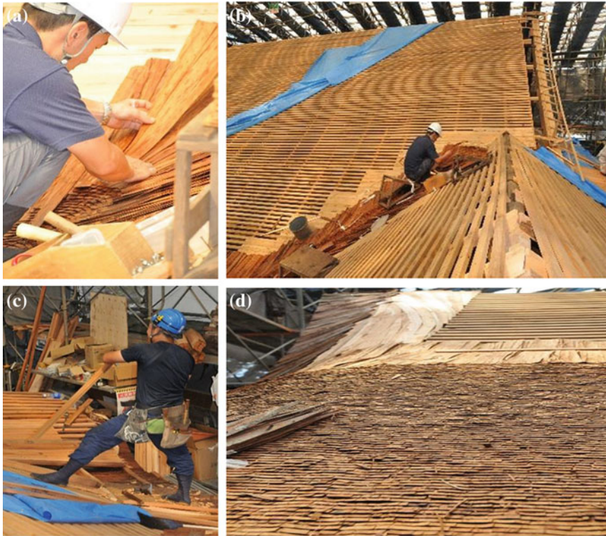
Fig. 6 (a-d) Cypress bark roof installation at Gekkodden pavilion. Hiwada contractors, specialised in cypress bark roofing, work in a team of four to five, commencing with the layering from the base of the roof line moving towards the top. Singular cypress strips are secured with small galvanised steel nails ( photographs by author )
